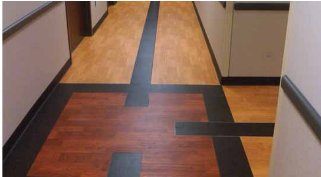
First floor renovation of the Iowa City Department of Veterans Affairs by Covenant Construction Services (hallway pictured)
