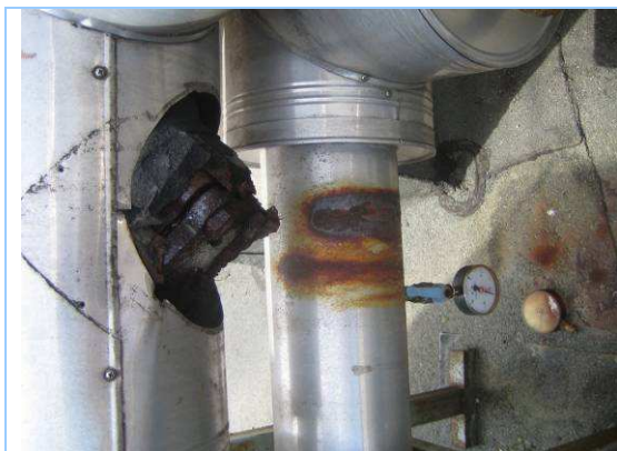
Figure – damaged insulation
