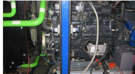
Figure – Equipment pictures
