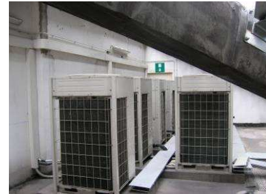
Figure – Equipment pictures
