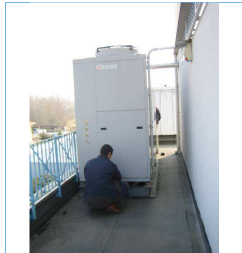
Figure – Equipment pictures
