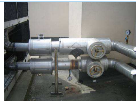
Figure – cool water inlet and outlet
