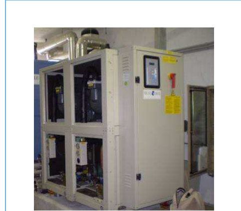
Figure – Equipment pictures
