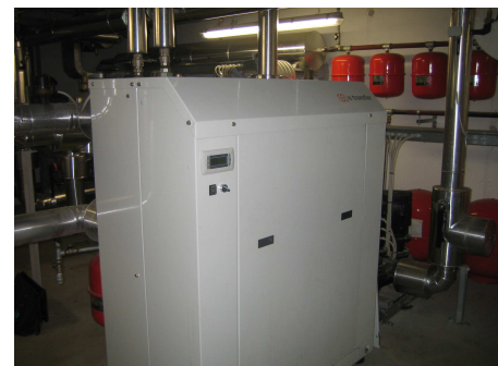
Figure – Equipment pictures
