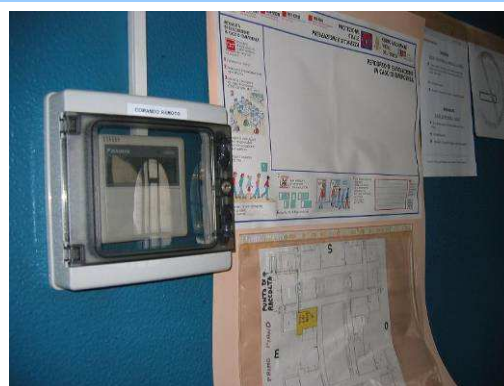
Figure – Control panel
