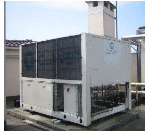
Figure – Equipment pictures
