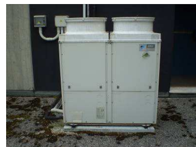
Figure – Equipment pictures
