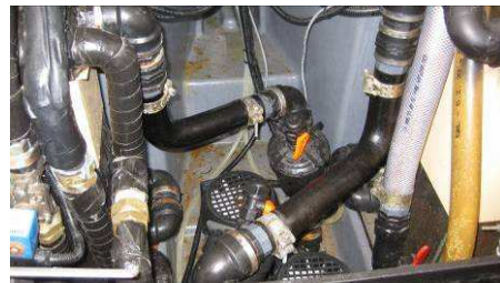
Figure – Li-Cl Solution pumps
