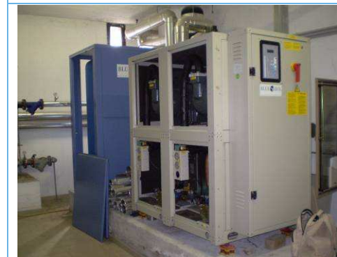
Figure – Cold generator Plant
