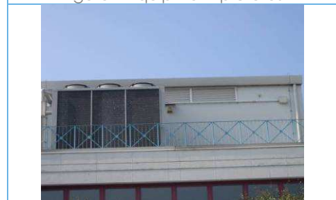
Figure – Cold generator Plant
