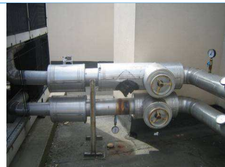
Figure – cool water inlet and outlet
