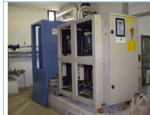
Figure – Cold generator Plant
