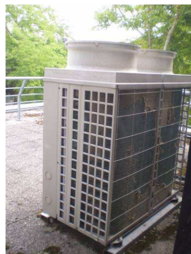
Figure – Equipment pictures
