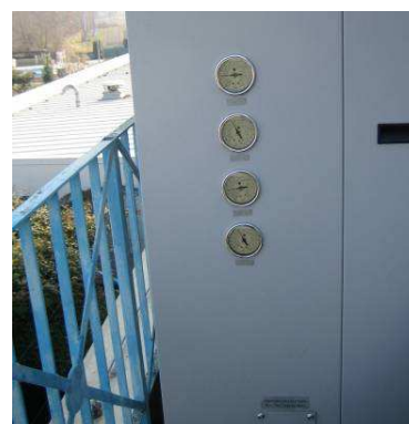
Figure – Pressure gauges
