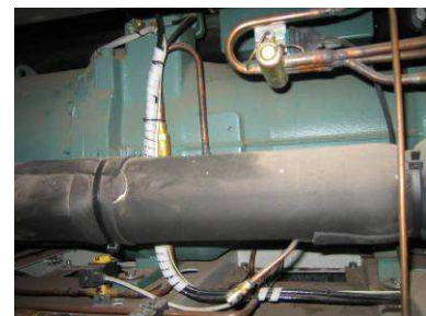
Figure – Equipment pictures
