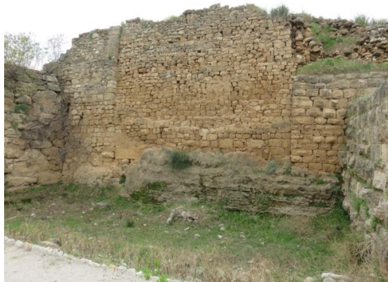
Figure 3.24: The retaining wall no.16 of the Persian Complex at Byblos, looking southwest (Photo by Author)
