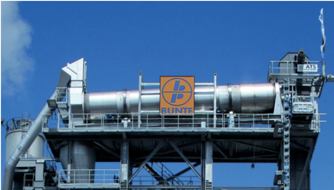
Fig. 2.32: parallel dryer installed on top of the Bunt batch plant
