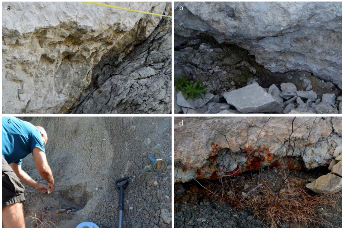
Figure 60. Clay-shales: a, b and d) at the contact with the rock slab; c) during the sampling in the northern area of the slab.
