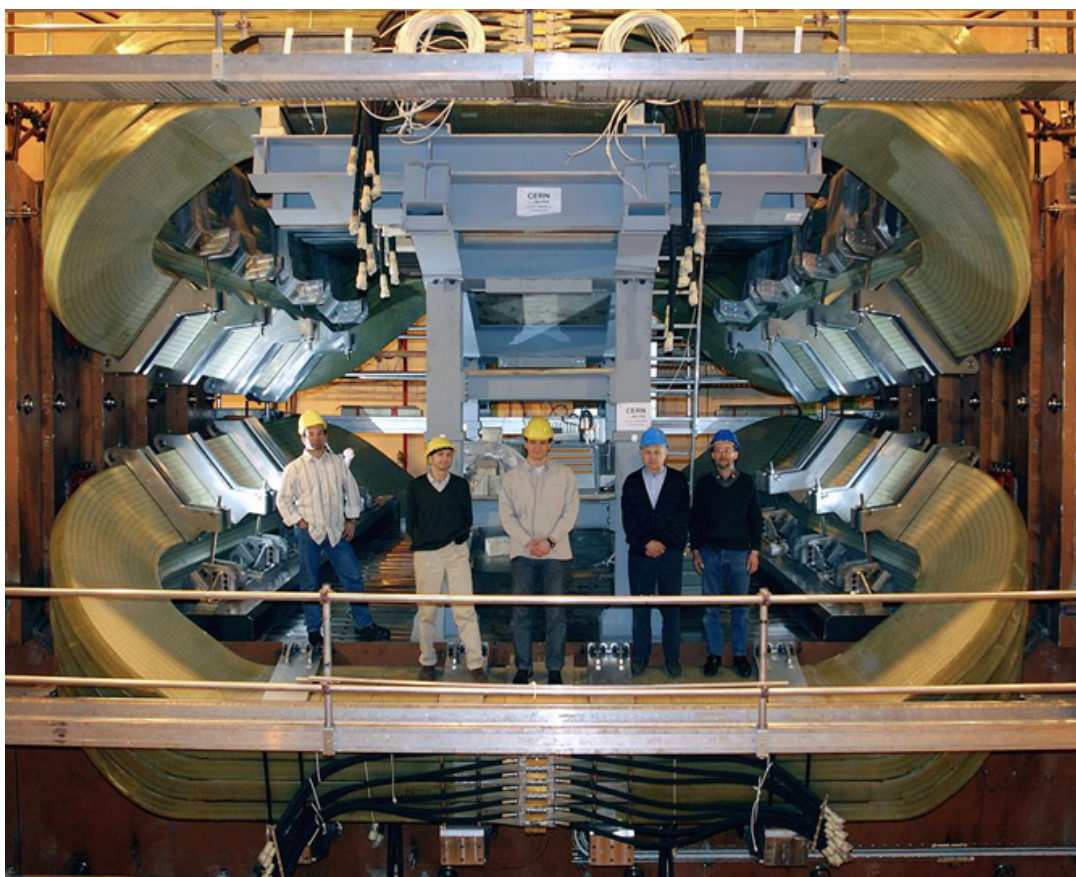
Figure 2.5: Front view of the LHCb dipole magnet after the installation in the detector cavern. The particular profile of the two coils, in order to follow the detector acceptance, is visible.
