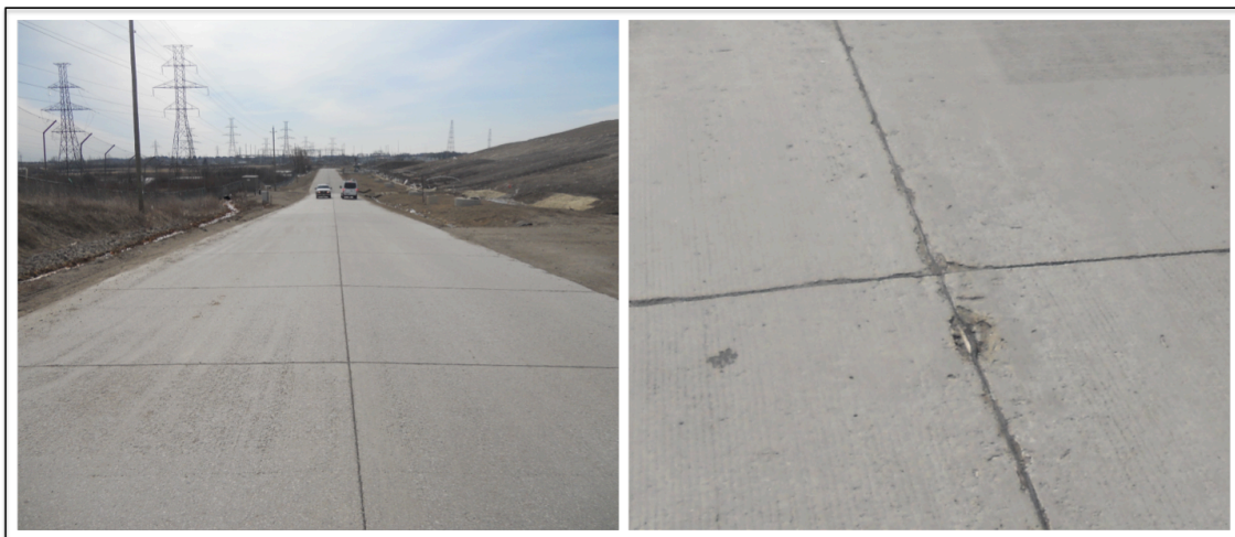
Figure 5.7: View of various distresses in the CPATT Test Track rigid sections.
