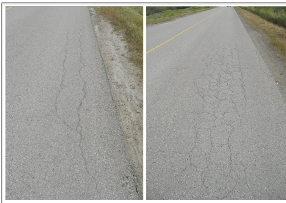
Figure 5.6: View of various distresses in the CPATT Test Track flexible sections.
