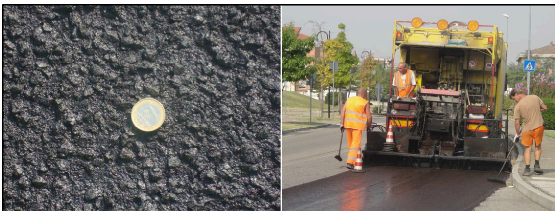
Figure 4.8 Close-up picture of the multipurpose microsurfacing (left) and construction phase in Ozzano dell'Emilia (right).
