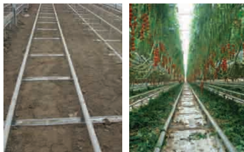
Plate 11 Pipe/rail heating systems
