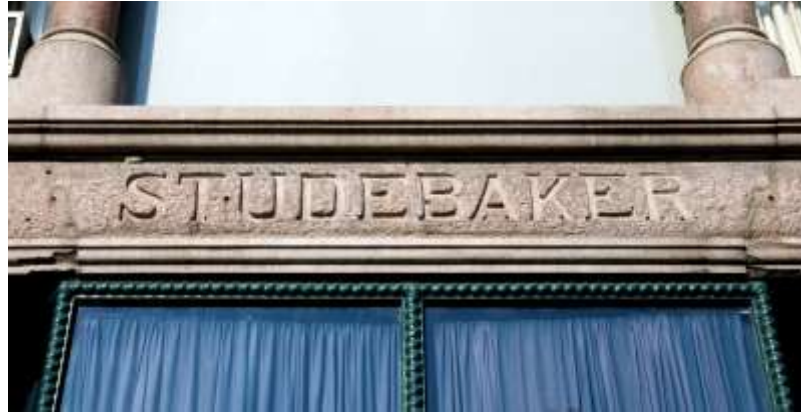
Figure 3.12 Solon S. Bemen & Irving K. Pond, Studebaker Building stone lintel joints (1884), photo by author.
