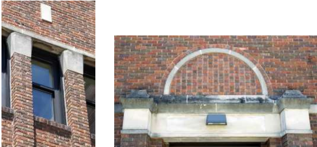
Figure 4.10 Claude & Starck, Mount Horeb Public School; window and stone capital (top), doorway detail (bottom). Photos by author.
