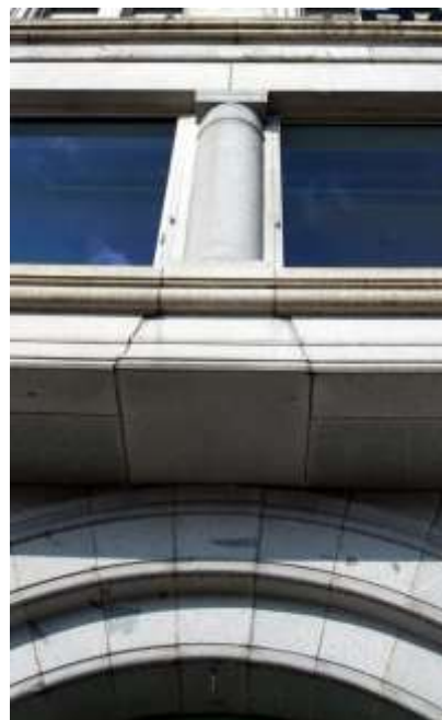
Figure 3.13 Adler & Sullivan, Auditorium Building stone lintel joints (1889), photo by author.
