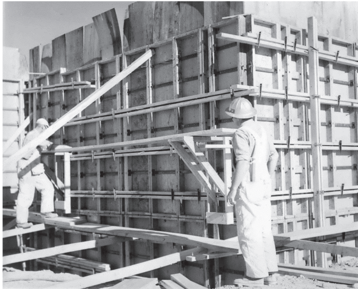
Figure 10: Plywood boards used in formwork to create the Shadowood texture of the walls. . Image Credit: Jackson Hole Historical Society
