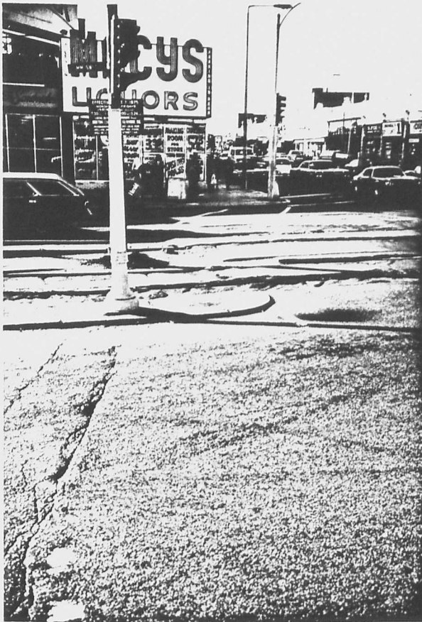
Figure 48. Lack of Signal Indications at Pedestrian Crossing, Commonwealth Avenue at Harvard Street
