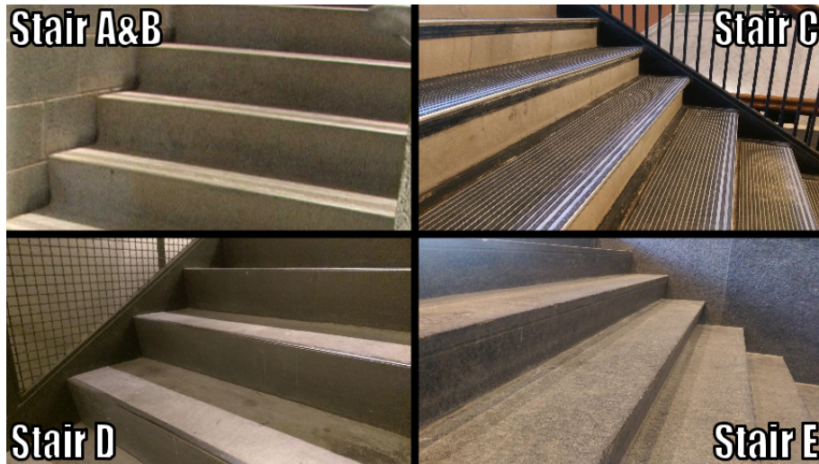
Figure 5. Stairs used to test the semi-autonomous behavior
