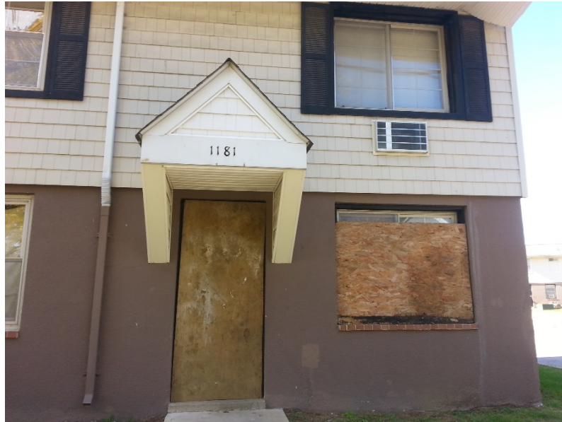
Figure 19. Eastport Terrace, vacant unit
