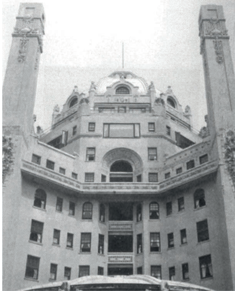
Figure 1. Detail of the concrete façade of the Blenheim building of the Marlborough-Blenheim Hotel in Atlantic City, NJ (1905). 16
