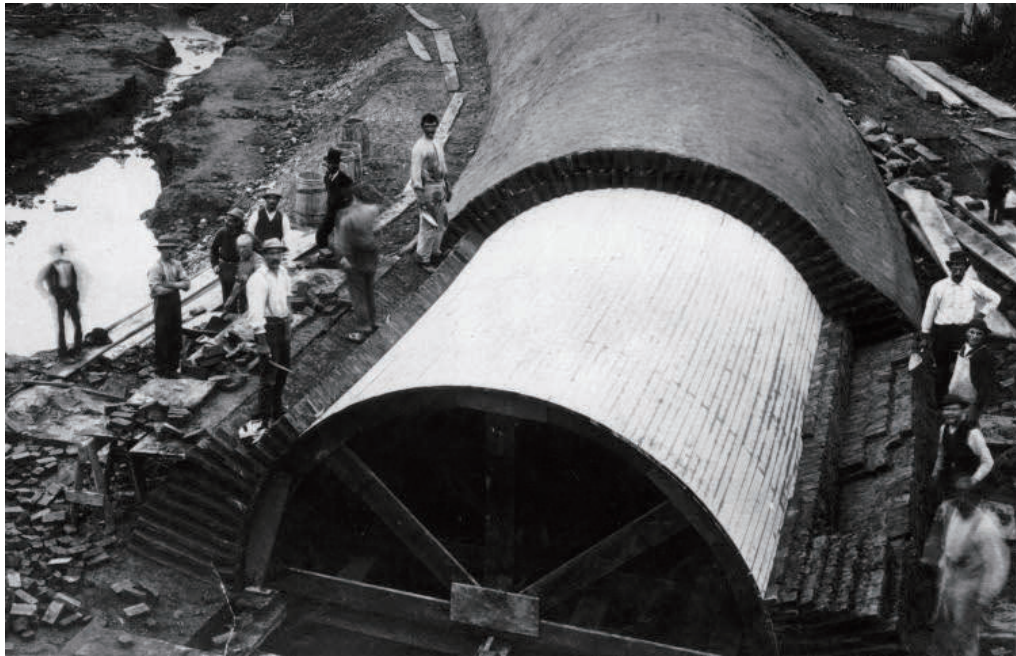
Figure 15: The Mill Creek Sewer in West Philadelphia, under construction. Photo Source: Philadelphia Water Department Archives
