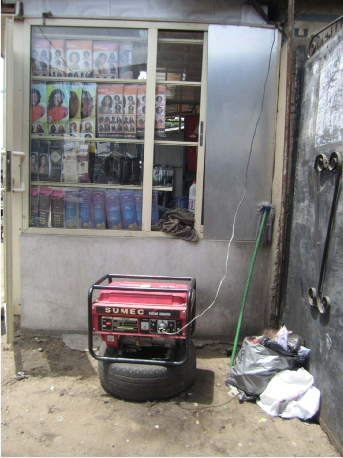
Figure 2: Generator powering Bubbles Salon
