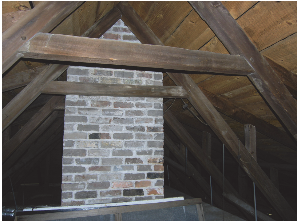
Figure 16. Present day photography illustrating heavy timber roof structure and masonry chimney. Image credit MCH.
