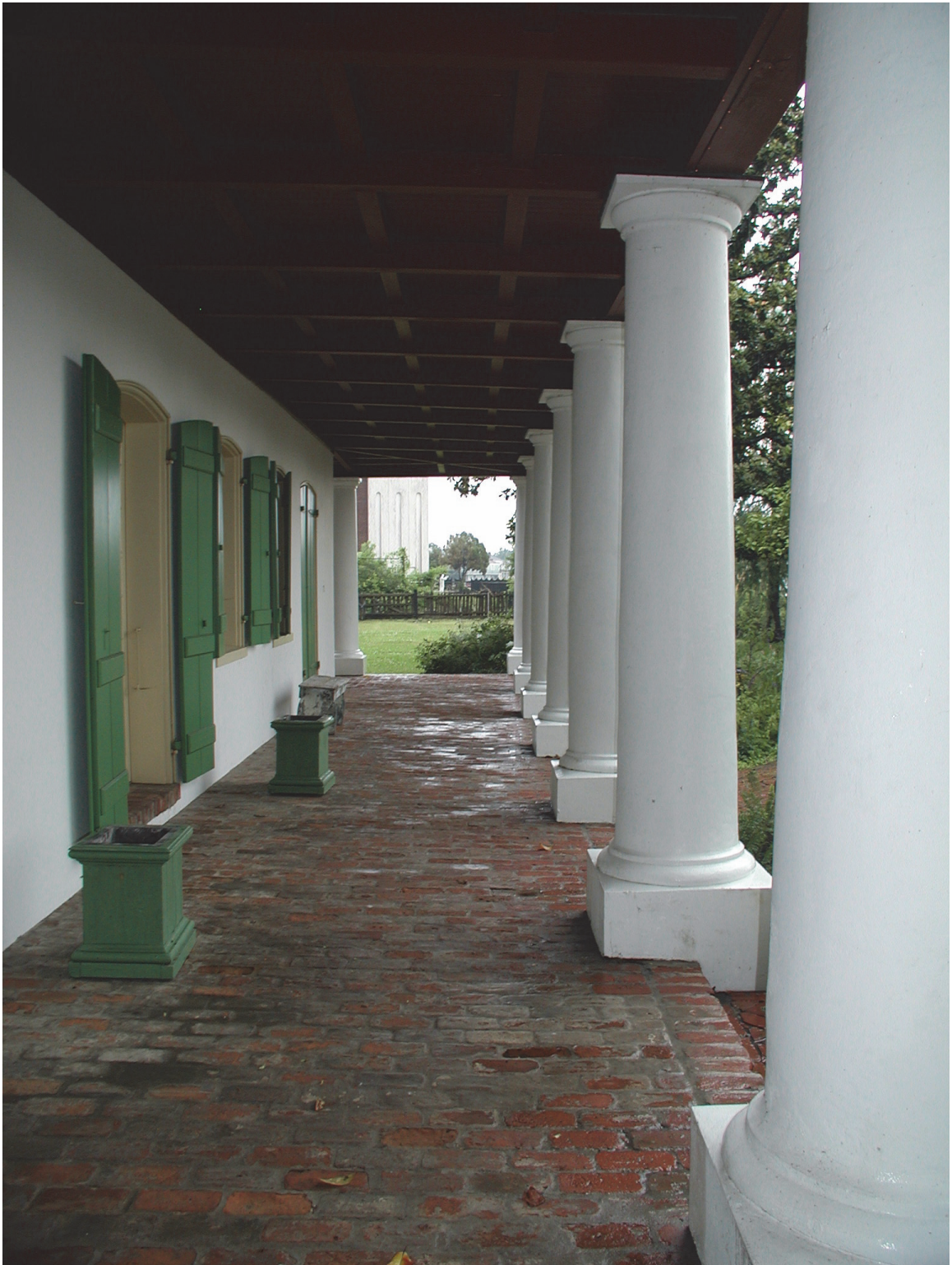
Figure 14. Present day photograph of the first floor gallery, note the masonry floors. Image Credit Michael C. Henry (MCH).
