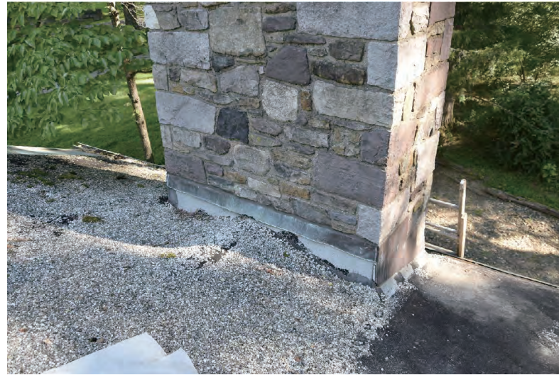
Deteriorated copper flashing in the chimney shaft base
