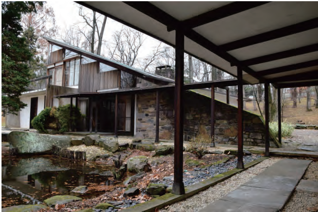
Fig. 4.4: South elevation view. Date: December 2014. Notice the new gutter system, the new ipe posts upon ipe bases, and the opaque white paint covering the plywood soffit. As shown in fig. 4.1, the concrete floor of the terrace has been waterproofed.
