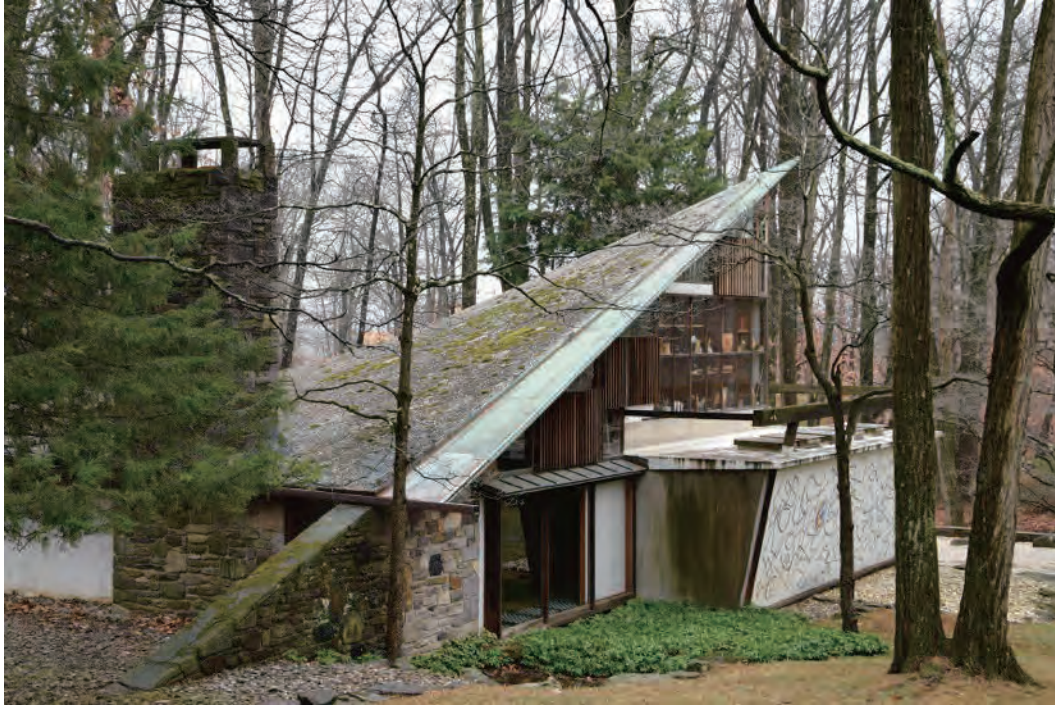
Fig. 4.2: West elevation view. Date: December 2014. Notice the new gutter system, the copper canopy, and the new skylights. The various copper patinas are indicative of new and old flashing campaigns. In addition, the concrete floor of the terrace shows a waterproofing coating painted in white, which disrupts the original aesthetic. Furthermore, landscape features have been changed over time. All photographs by César Barges Ballester, unless otherwise noted.
