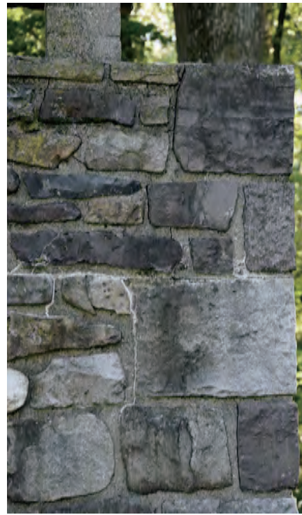
Right corner, closer view of deteriorated bed joint, mineral accretions, and cracks
