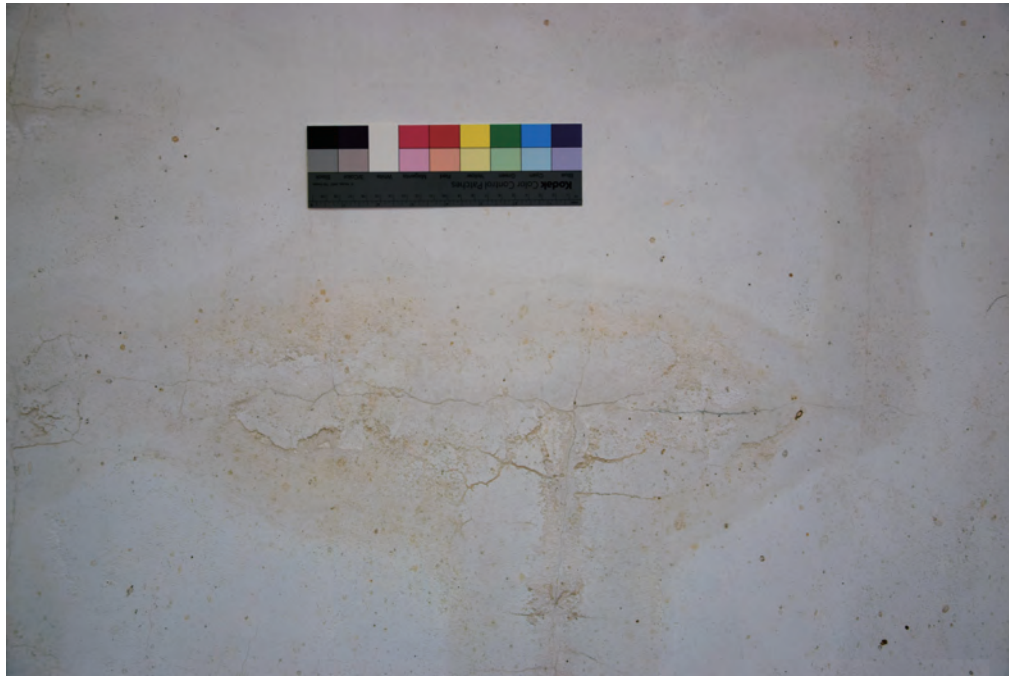
Fig. 5.1. This picture shows wet moisture stains along with hairline cracking map, efflorescence, superficial erosion, and light brown mineral deposits filling the cracks.
