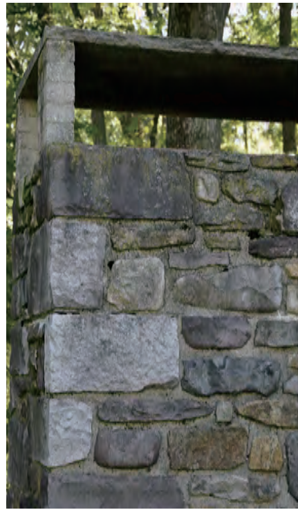
Left corner, closer view of deteriorated bed joint
