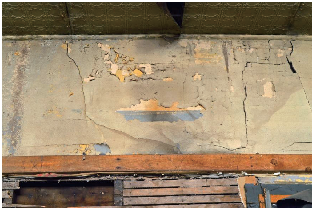
Figure 3.29 Loss of plaster and most recent finish on middle section of south wall (Author 2014).
