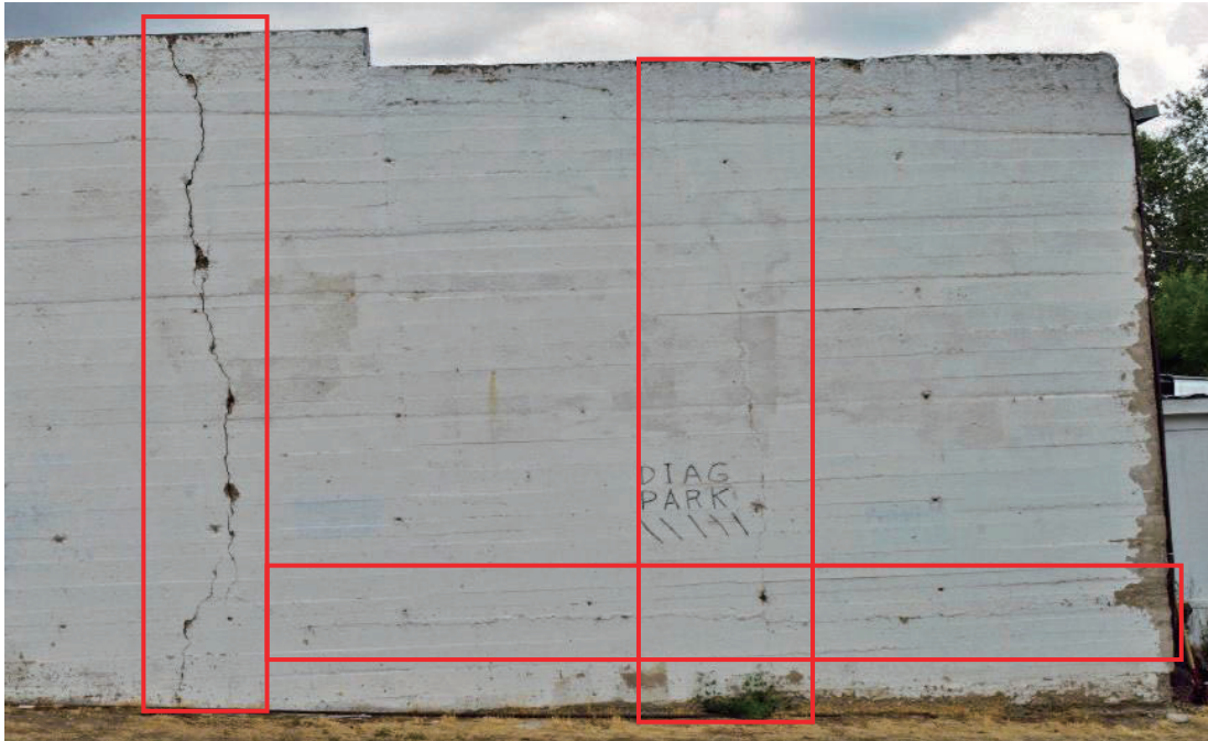
Figure 3.7 Southern portion of exposed west wall with cracks highlighted (Author 2014).
