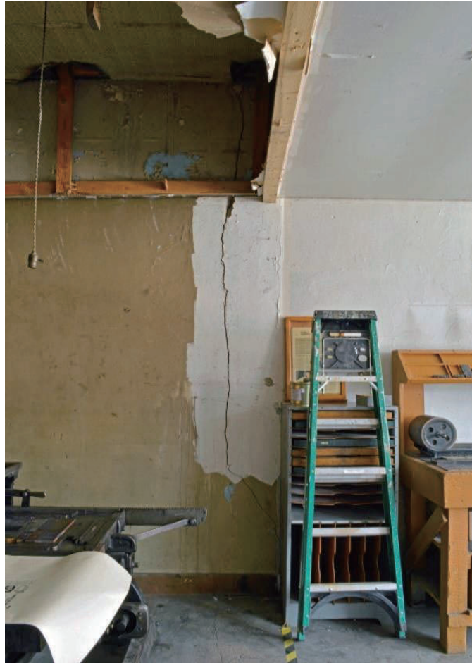
Figure 3.8 Primary crack on west wall seen from the interior (Author 2014).
