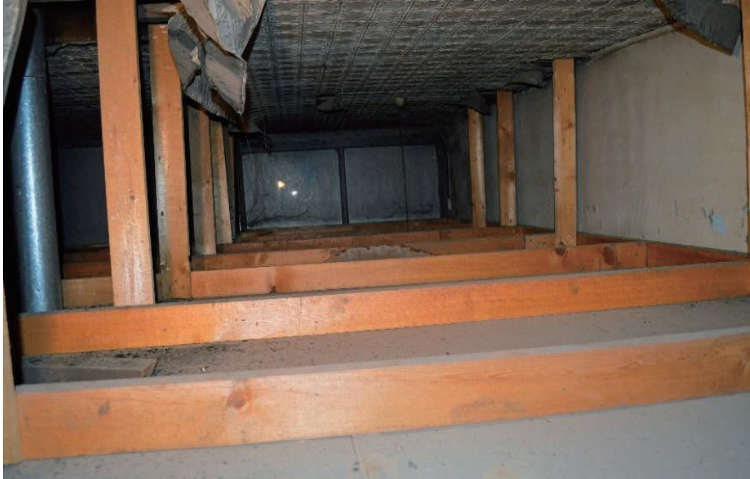
Figure 3.23 Northern view of the space between the drop ceiling and the pressed metal ceiling (Author 2014).
