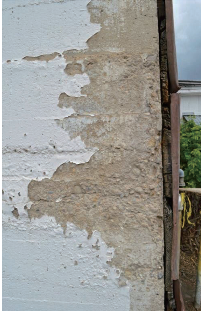
Figure 3.6 Weathering on southern edge of exposed west wall (Author 2014).
