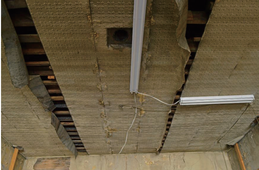
Figure 3.25 Peeled back pressed metal ceiling for removed drop ceiling supports and cut rectangle for removed stove (Author 2014).
