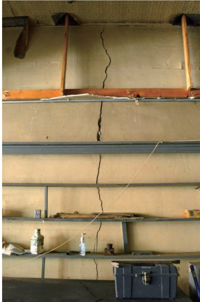
Figure 3.10 Crack on east wall seen from the interior (Author 2014).
