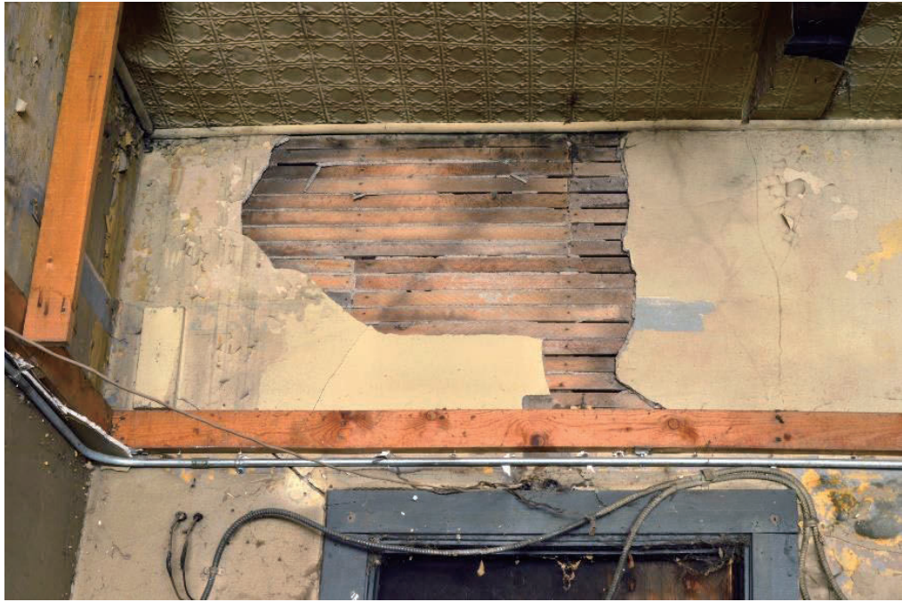
Figure 3.28 Plaster loss above east window on south wall (Author 2014).
