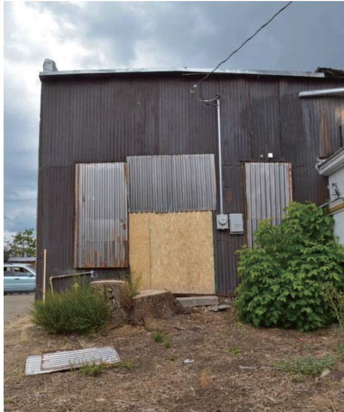
Figure 3.3 Stump of tree compromising the foundation and floor (Author 2014).
