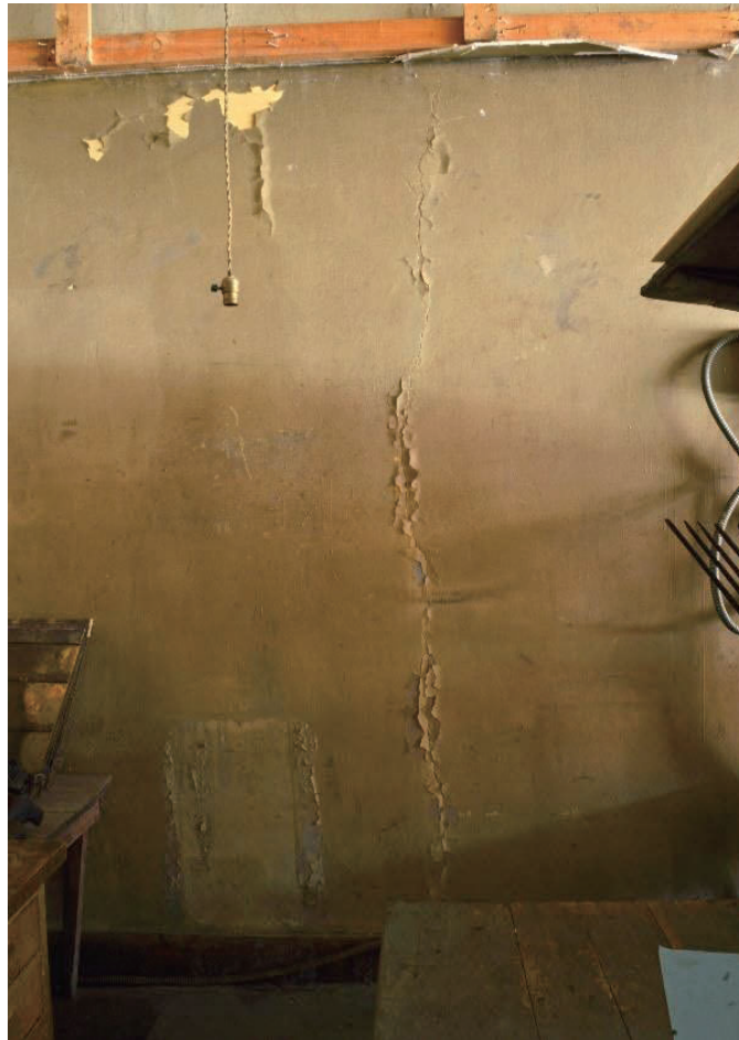
Figure 3.9 Secondary crack on west wall seen from the interior (Author 2014).
