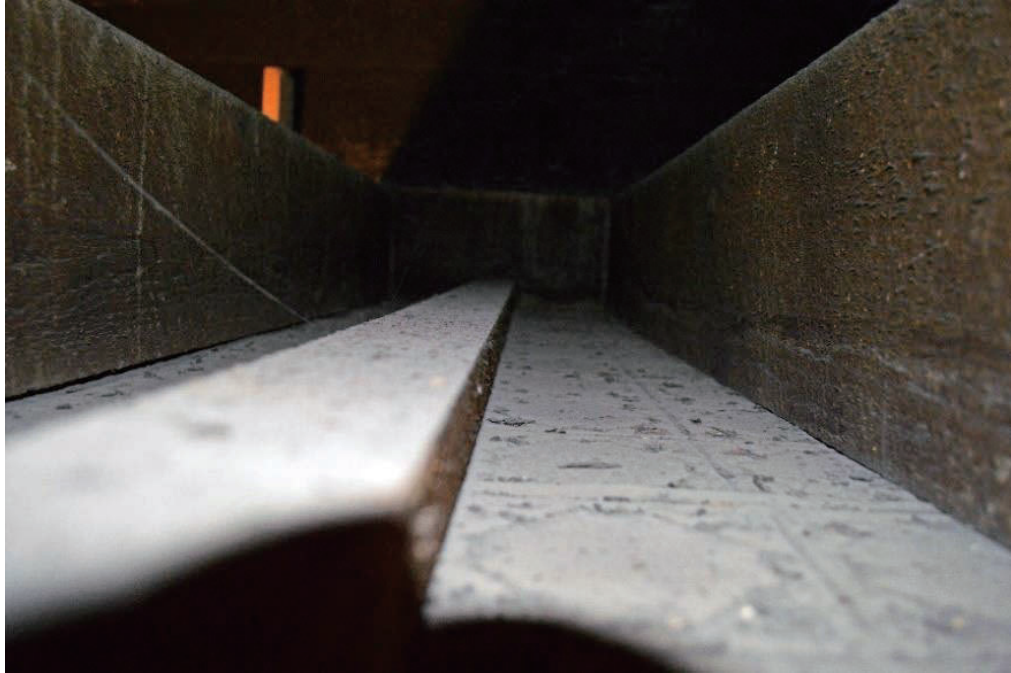
Figure 3.21 Underside of pressed metal ceiling fastened to horizontal rafters and nailers (Author 2014).
