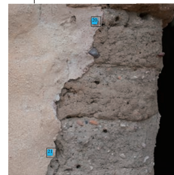
TUMA_20 Pink repair directly on rebuilt adobe TUMA_21 Pink repair directly on rebuilt adobe
