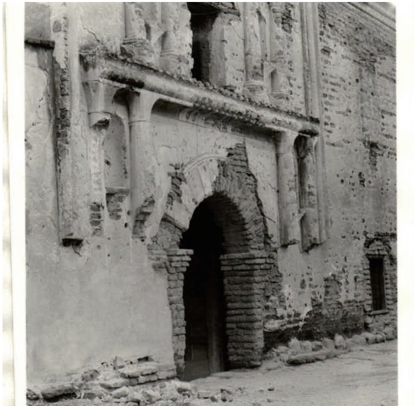
Figure 5.1: Photograph indicating damage from 1944 storms 22
