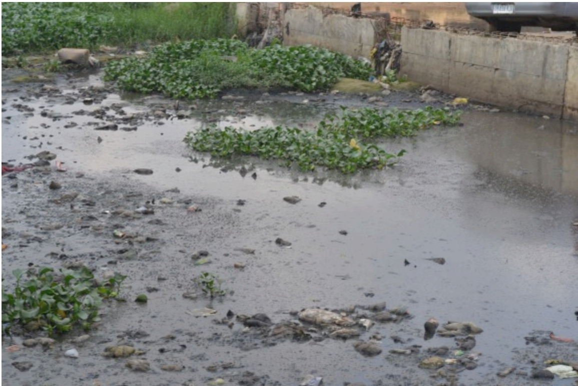
Figure 9: Polluted & Blocked Canal
