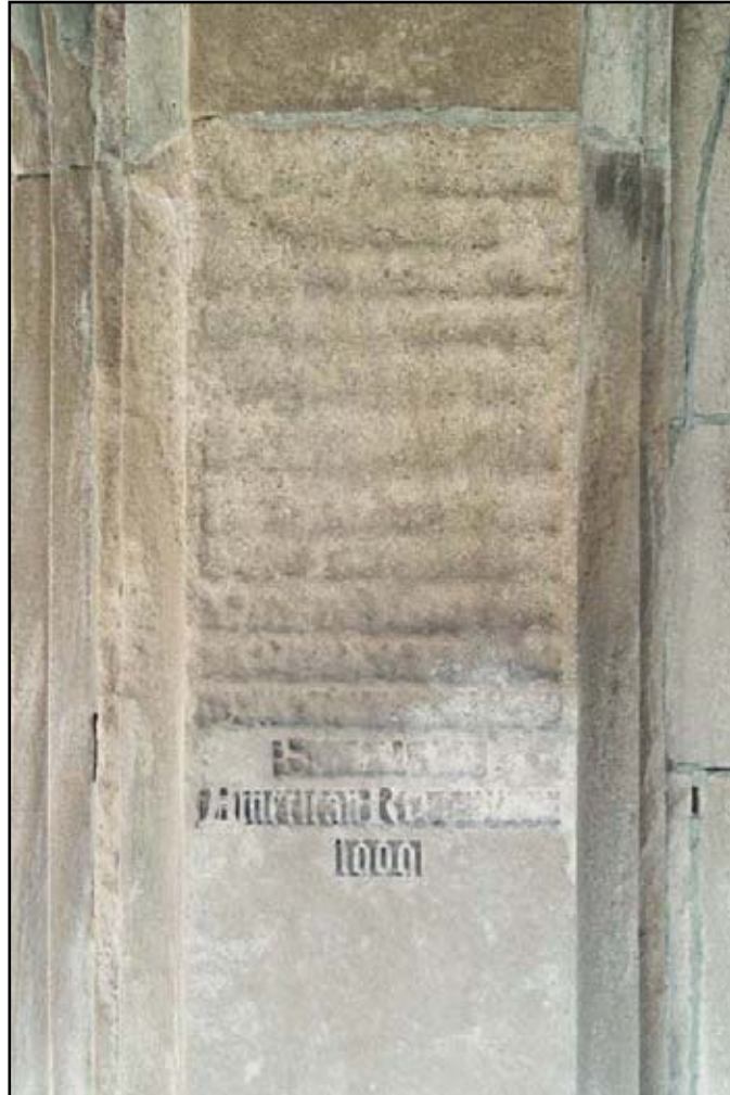
Figure 58. Area below a leak in the Cloister roof, which is allowing rainwater to erode the stone's surface.
