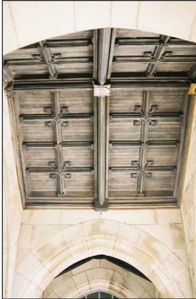
Figure 14. The cloister roof is constructed of Indiana white oak in a tongue and groove pattern and supported by bevel edged trusses.
