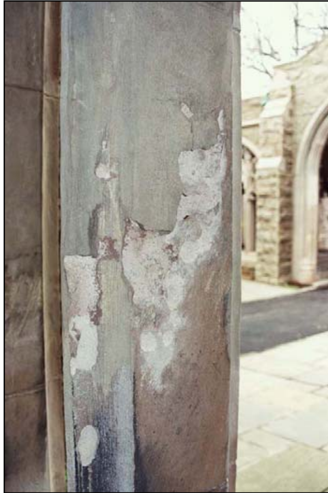
Figure 56. Delamination of the stone presumably caused by salt crystallization.
