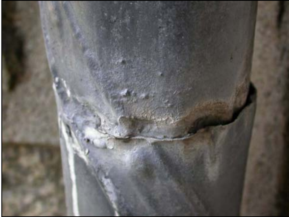
Figure 63. Joint repair & corrosion on downspout located on west façade, south end.
