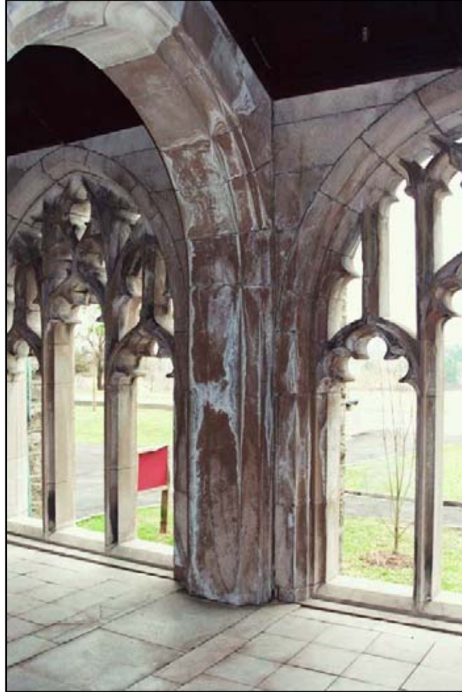
Figure 55. Salt efflorescence in the Cloister of the Colonies.
