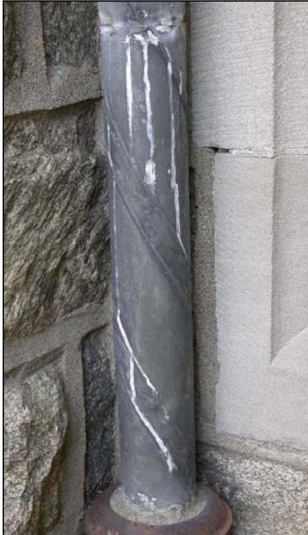
Figure 64. White corrosion drips on downspout on west façade of the Cloister, southern end.
