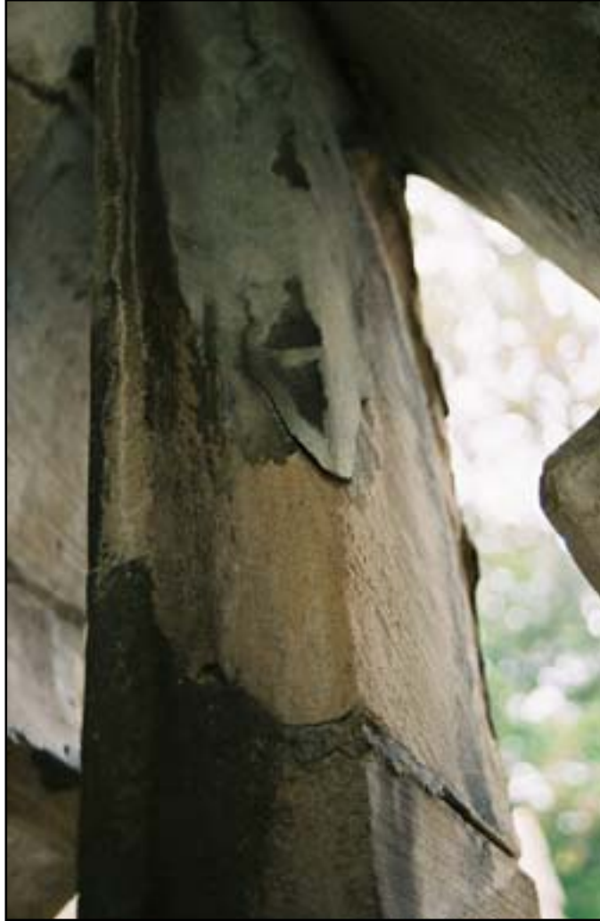
Figure 57. Cement patching separating from the limestone body.
