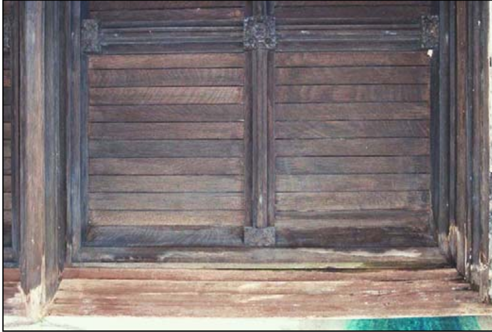
Figure 61. The oak ceiling is exhibiting water damage in small areas due to the leaking roof.
