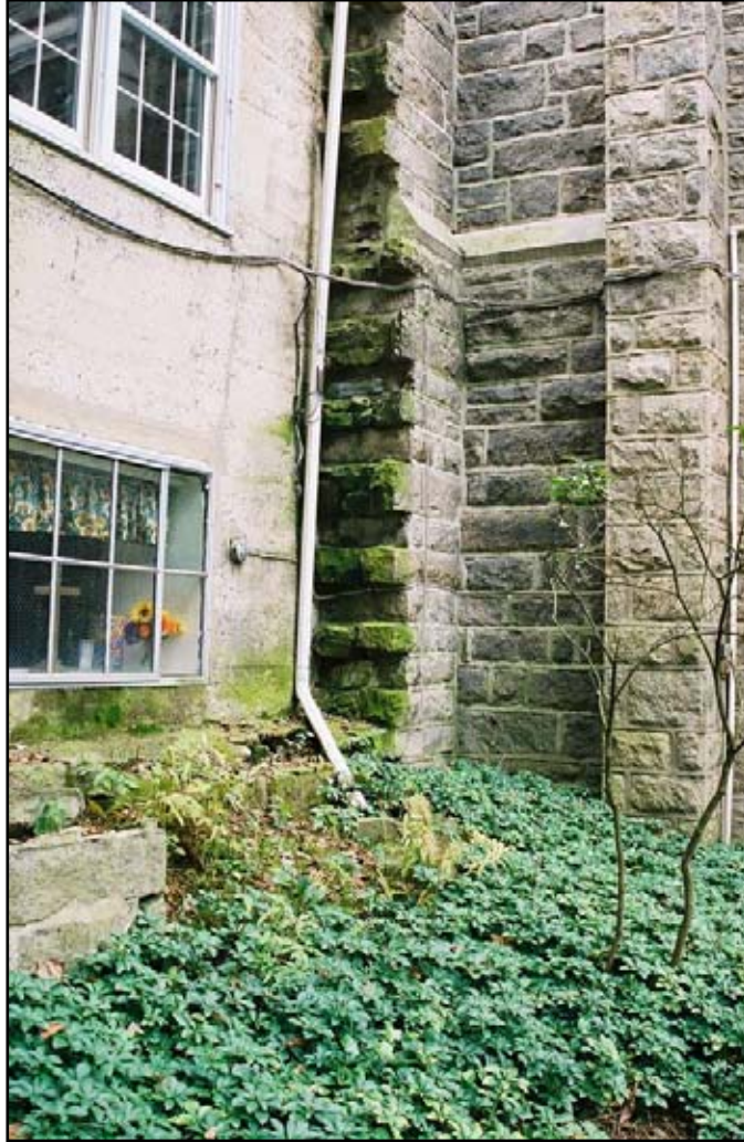
Figure 53. Biogrowth attacking the damp stone and stucco on the north wall of Patriot's Hall.
