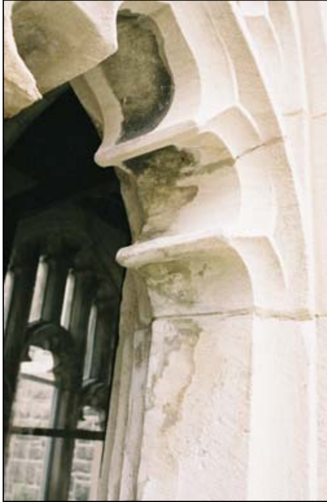
Figure 60. Black staining is found in areas that are not washed by rainwater.
