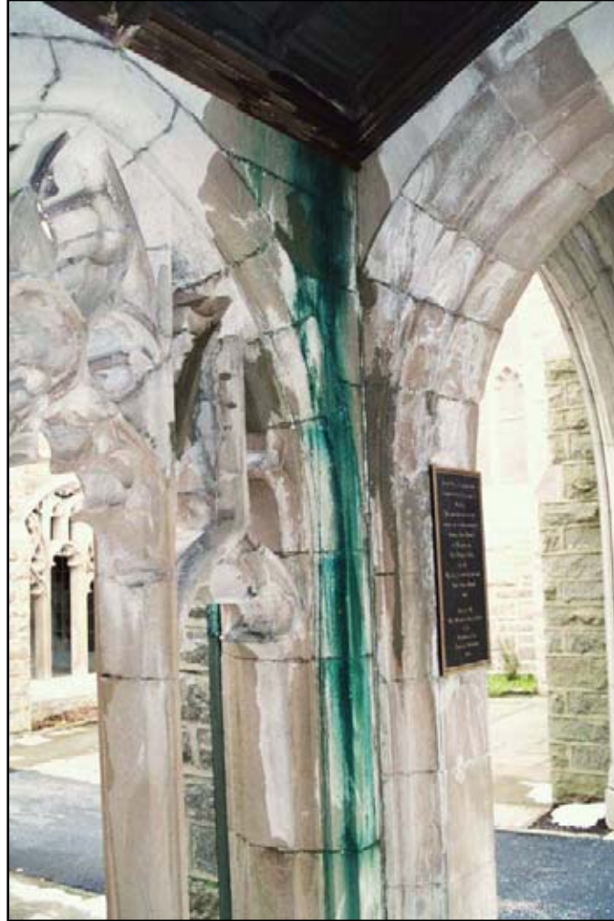
Figure 59. Copper staining from the Cloister gutters is spreading below a leak in the roof.
