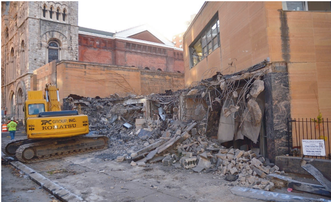
Figure 9 | Demolition scene of the Hillman Medical Center. Source: Ben Leech, Hidden City Philadelphia , 2011.
