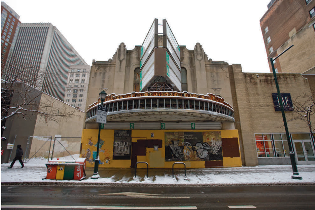
Figure 4 | The Boyd Theater days before the demolition began on its interiors. Source: Bradley Maule, Hidden City Philadelphia , 2014.
