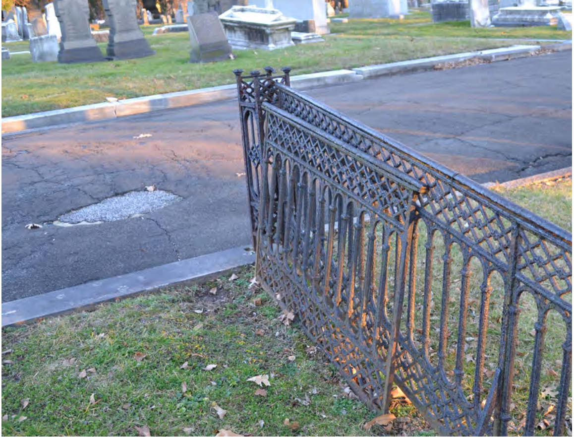
Figure 2.8. Dislodged and corroding front fence panel.
