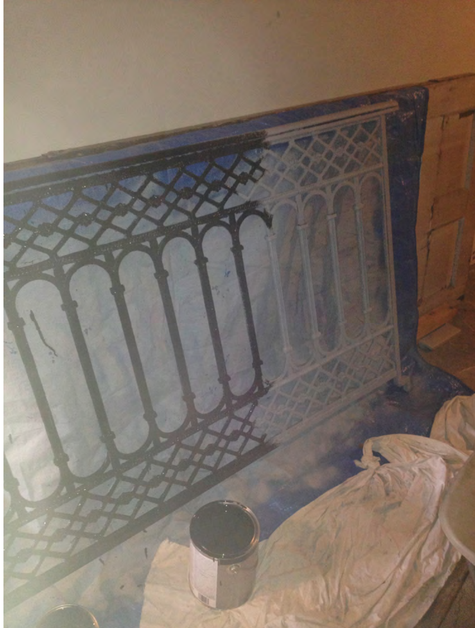
Figure 2.11. Fence panel midway through first coat of oil based paint application. The white portion of the fence shows the corrosion inhibition primer application.
