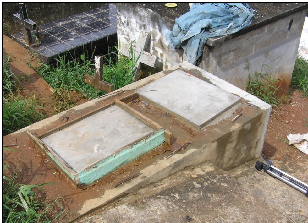
Figure 6-9. Cement slabs used to seal tombs are being constructed on the top of SCS CAT 774 (photograph by C. Fellows).
