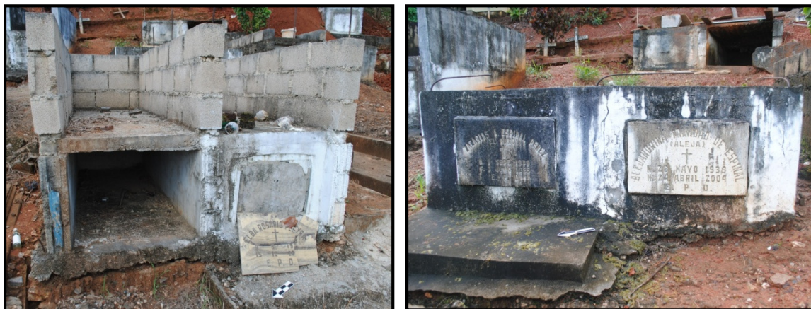
Figure 6-8. On the left is SCS CAT 32, which displays a second level that is currently under construction. Note the cinderblock structure. SCS CAT 25, on the right, demonstrates the rebar protruding out of the tomb, which will later be used in the addition of a second level. Note that the rebar has been folded over (photographs by author).
