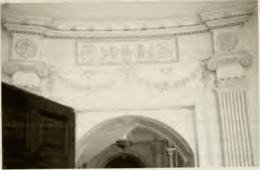
FIGURE 3.2.12 West door surround detail and door panel profile in the Oval Drawing Room. Photograph and drawing by author.
