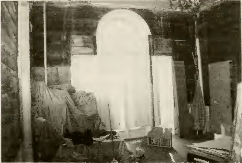
FIGURE 3.3.2 1997 Existing conditions in the Southeast Parlor after removal of gypsum drywall. South elevation (top) and North elevation (bottom). Photographs by author.
