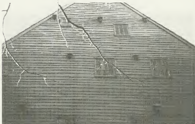
Figure 4: Exposed Beam-ends with Protective Shingle Covers
