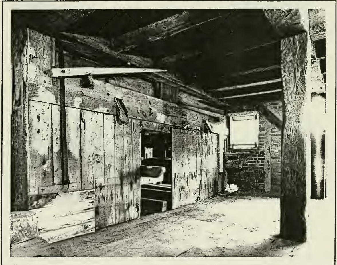
Fig. 32 Interior view of southwest corner, with the enclosed gears. The mechanism controlling the distance between the stones is operated by the lever in the top left corner. (HAER NY-106-11)
