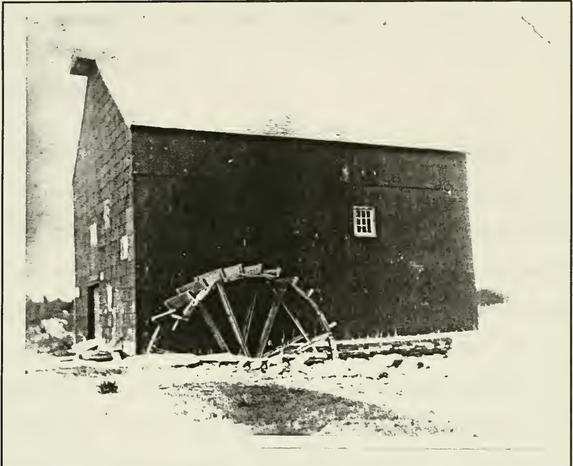
Fig. 27 The mill with its wheel still intact but badly damaged, southwest elevation. (HAER NY-106-19)
