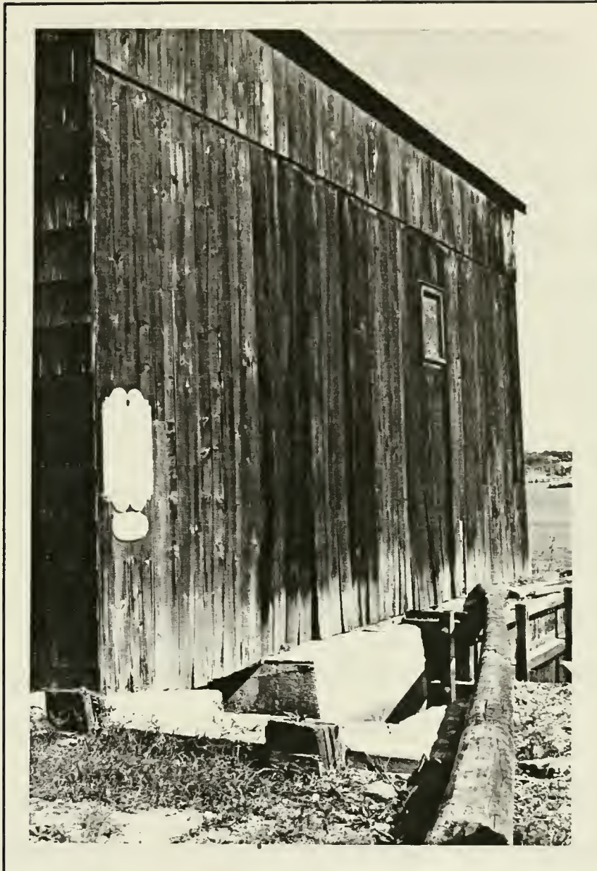
Fig. 38 Badly deteriorated wood sidings, south elevations. Also notice the original location for the water wheel.
