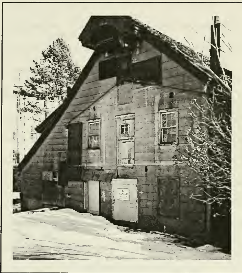
Fig. 18 Roslyn Mill, general view from the back. Advanced deterioration showing, as well as changes that were done to the facade.
