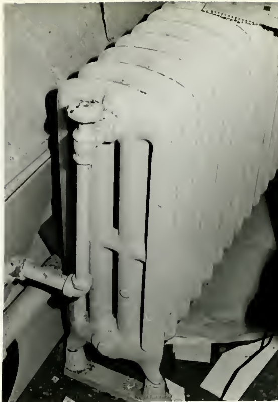
ILLUSTRATION #21 - Radiator located in second floor addition studio above main reading room. This type of radiator is typical of a type manufactured after ca. 1910 and is located in a section of the building which was not original to the building, thus it is certainly not a part of the original steam heating system.
