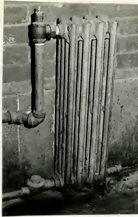
ILLUSTRATION #23 - Radiator located at the first floor of the stair tower near the entry to the library. This radiator is typical of segmental cast iron radiators which were manufactured circa 1900.
