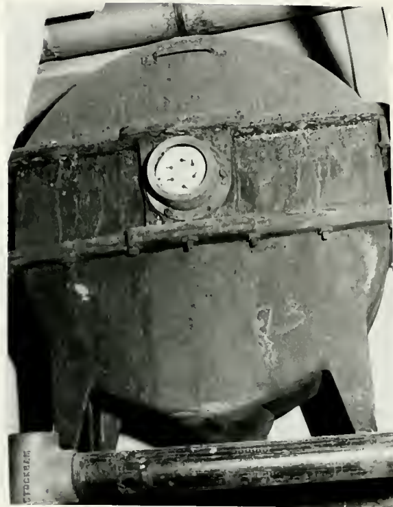
ILLUSTRATION #28 - Condensation meter found in the mechanical room for the building. This condensation meter, which measures by returning condensation the amount of steam used in the library heating system, was manufactured by the Central Station Steam Co..
