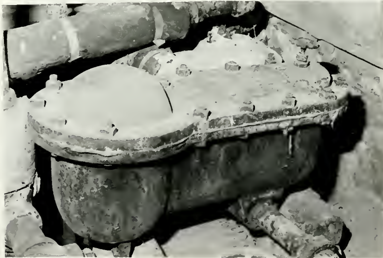
ILLUSTRATION #26 - Steam trap located in the mechanical room for the building. This type of "float" steam trap is imprinted with "No. 2, McDaniels Special Steam Trap, Patented Aug 19, 1890."
