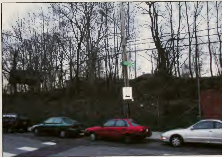
Figure 51 A chain link fence replaced the perimeter brick wall on Banbridge Street between Taney Street and 26th Street.
