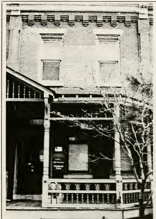
Figure 8. 628 Benson Street Camden, NJ. Inappropriate repointing on the front elevation of the building.
