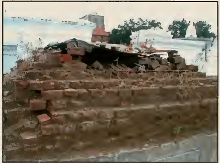
Fig. 4.12 Failed flat roof on a platform tomb.
