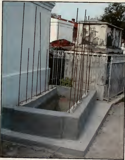
Fig. 2.8 Tomb #475, A Perpetual Care tomb being rebuilt, replacing the original historic materials.
