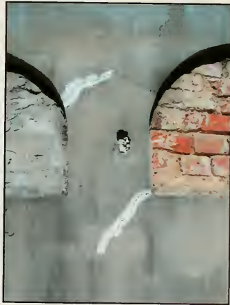
Fig. 6.26 The cement encasing the oldest section of wall vaults is cracking and has been poorly patched.
