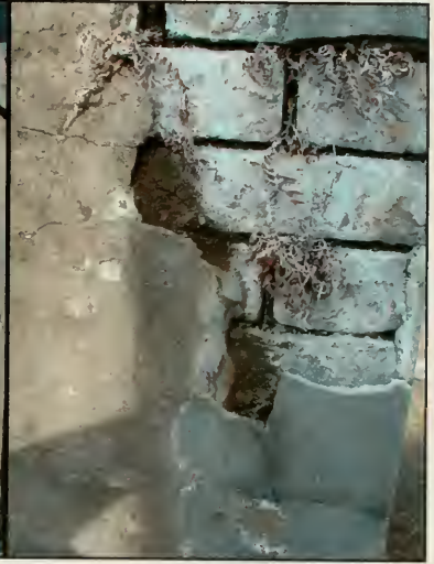
Fig. 4.6 Open mortar joints and evidence of wetness
