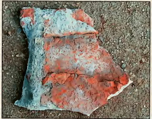
Fig. 3.15 Brick fractured by cement stucco. This is a sample from Tomb #275 where a new layer of cement stucco had been applied directly to the brick in locations where the old stucco had delaminated.
