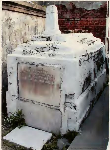
Fig. 6.21 Thick layers of peeling modern surface finishes, incomplete coverage and excessive biological growth in all the cracks and openings. Studio photograph, March 2001.
