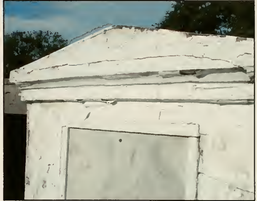
Fig. 4.3 An example of cracked and peeling modern finish..
