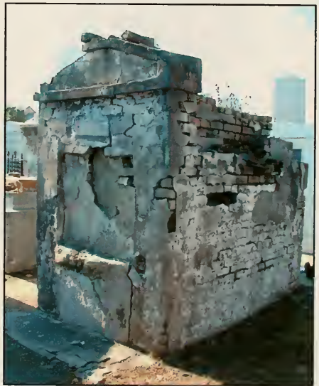
Fig. 6.16 Tomb #39, an example of years of deferred repairs. Periodic patching with cement and modern paint over the failing structure has provided no benefit.
