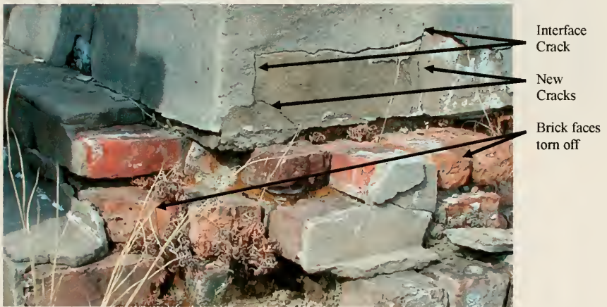
Fig. 6.10 Tomb #558 was originally covered in Tan stucco and has been patched with Gray (cement). When the Gray layer failed, it cracked at the interface with the original stucco, forcing new cracks into that layer, and tore off the brick faces wherever it was directly adhered. In some cases the released stress caused the pulling out of the entire brick. The missing bricks in the image above were found on the ground about the tomb with the cement stucco still firmly attached.
