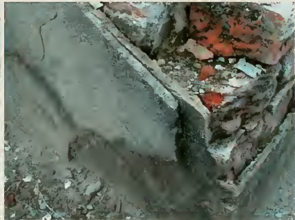
Fig. 6.4 Tan and Gray stucco layers evident.
