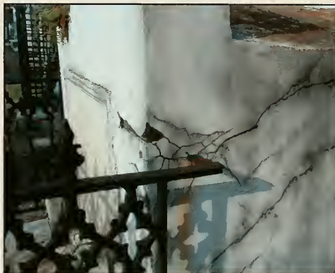
Fig. 4.13 Tomb #14, Cracking at the interface of stucco and metal connection.
