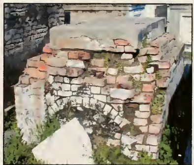
Fig. 6.19 The stucco has been completely breached. Mortar has been replaced by moss. Studio photograph, March 2001.
