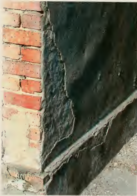
Fig. 4.4 Delamination and deformation of Stucco
