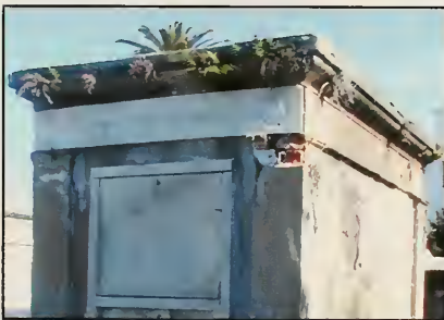
Fig. 6.18 Bio-film and moss have progressed to high level vegetation. Ferns are growing in the roof cracks and will soon cause major destruction. Studio photograph, March 2001.
