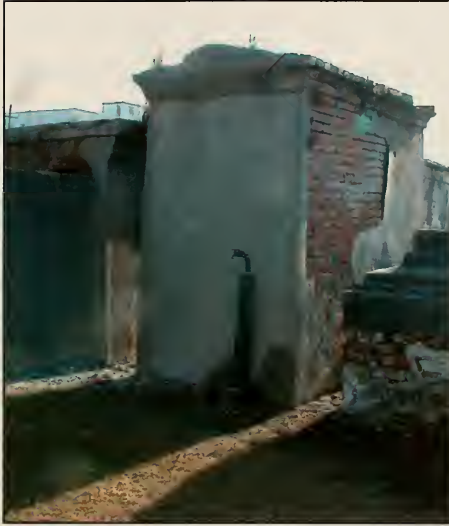
Fig. 6.8 The back of Tomb #600 covered in cement stucco. The front of the tomb is patched. Note the loss of the cornice with the new cement.
