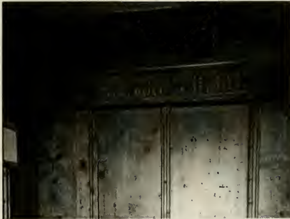
Figure E49. Swiss Room. Eastern portion of the south Engadine wall. Note smoke damage. (See page 57.)
