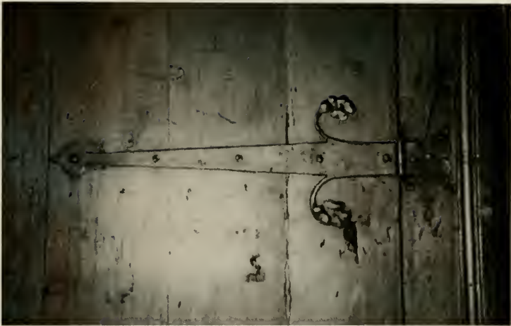
Figure E23. Swiss Room. Detail of the hinge on non-functioning door on the western section of the south Engadine wall. (See page 38.)
