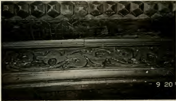
Figure E7. Swiss Room. Detail of Tirolean north wall. Note traces of gold paint remaining in the recesses of the carved relief of the molding. (See page 32.)
