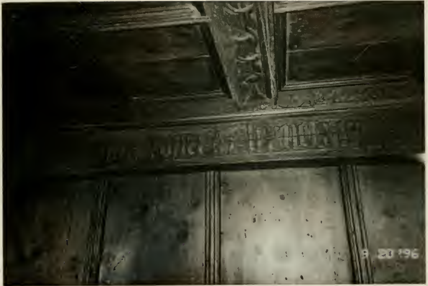
Figure E5. Swiss Room. Detail of north Engadine wall. Note the inappropriate separation of the moldings and batten by the wall plate. Also note the joint between the original molding on the right and the 1930s infill on the left. (See page 32.)
