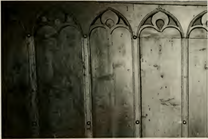
Figure E19. Swiss Room. Detail of the north Tirolean wall. Note the large, regularly placed studs used to hold the battens, friezes, and panels together. (See page 36.)
