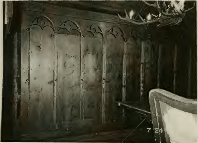
Figure A4. The Swiss Room looking west at the Tirolean wall. Note the chair rail line worn into the paneling. (See page 55.)
