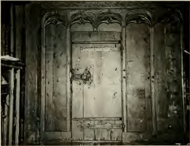
Figure E48. Swiss Room. East wall of Tirolean portion. Note abraded surface of panelling revealing wood borer damage, especially on the lower portion of the corner posts and the full length of the right corner. (See page 57.)
