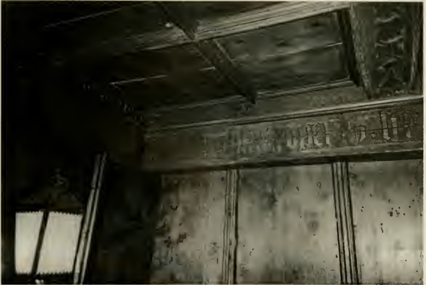
Figure E33. Swiss Room. Southwest corner of the Engadine section. Note modern coffered ceiling juxtaposed with exposed central heavy timber ceiling support overlaid with an Engadine molding. Also note exposed heavy timber wall plate with overlaid Romansch inscription. (See page 39.)
