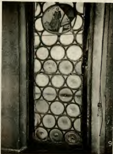
Figure E53. Swiss Room. Second easternmost lite in bay window. Note cracked roundels and broken comes. (See page 62.)
