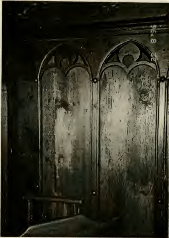
Figure E51. Swiss Room. The two westernmost panels of the north Tirolean wall. Note water damage due to the long-term placement of a coffee maker. (See page 58.)
