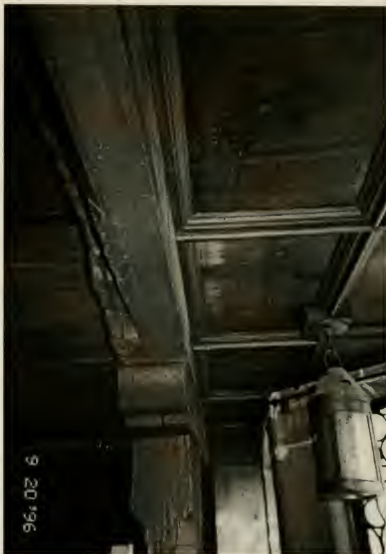
Figure E50. Swiss Room. Ceiling of bay window looking east. Note water damage from burst pipe. (See page 57.)
