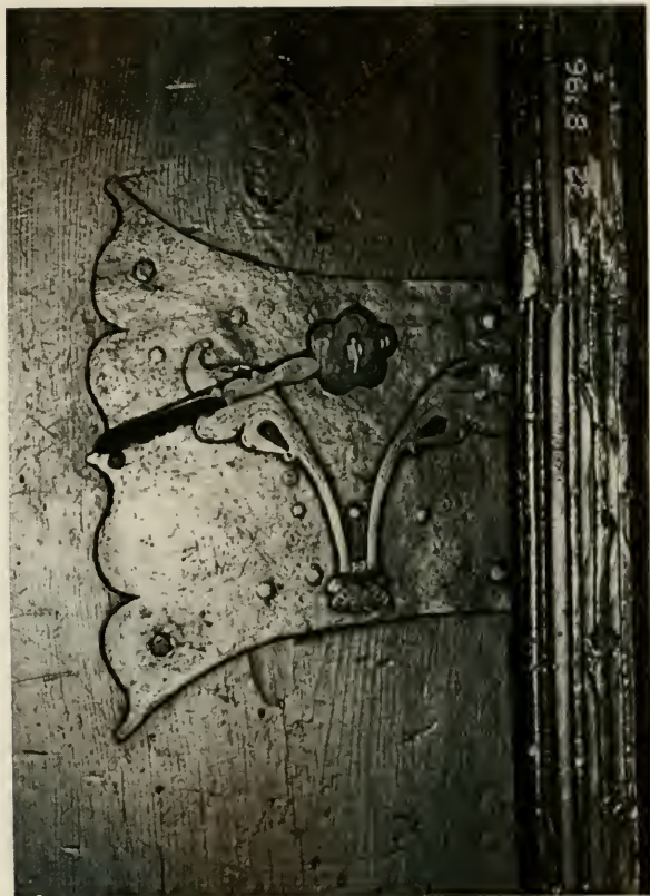
Figure E26. Swiss Room. Detail of latch and keyhole plate on the interior of the entrance door. Note multiple generations of attachments. Compare overall shape to Figure E27 and lock ornament to Figure 28. (See page 38.)
