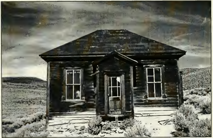
Figure 3.12a. Photo showing chemical failure of wood. Discoloration along bottom of wall due to black rot. Rm. 2, West wall, Selhorn taken 29, July, 1997 by P.D. Schulz. Figure 3.12b. Photograph of “weathering” of wood. East Elevation of McDonald taken 3 Sept., 1998 by A.S. Morrison.
