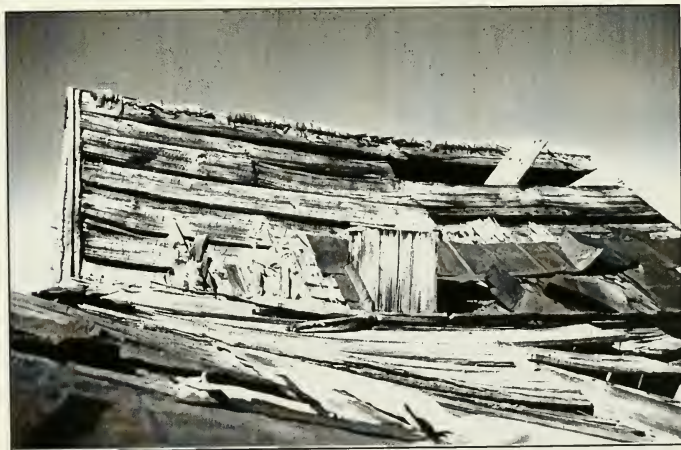
Figure 3.9a. Photograph illustrating deformation of "L" additions due to lateral loads. South-West Elevation, Building "D" taken 2 Sept., 1998 by A.S. Morrison.
