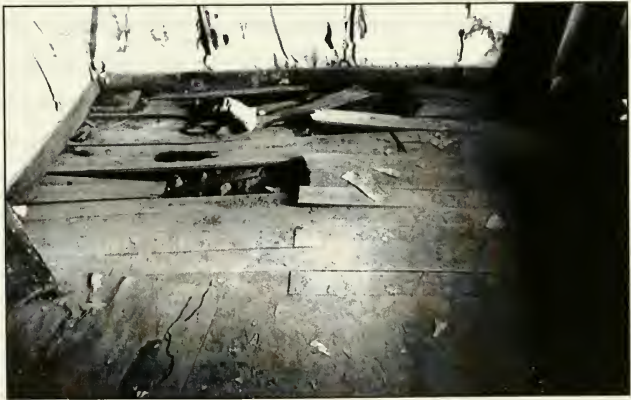
Figure 3.4a. Photo illustrating Tilt. Building O Privy taken 22 Sept., 1995 by P.D. Schulz. Figure 3.4b. Photo illustrating Heaving. Murphy, Rm. 4 taken 30 April, 1997 by author.
