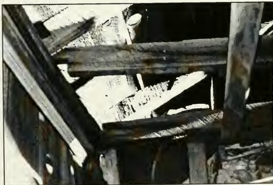
Figure 4.3a. Diagrams of intervention strategies for broken joints. Figure 4.3b. Photograph showing failure of connection. Bldg. "P" Rm. 1, NW corner taken 6 Aug., 1996 by P.D. Schulz.
