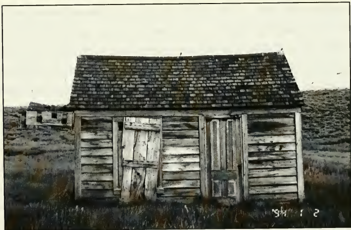
Figure 4.6a. Recycled tin can shingle w/ trademark blown off sheathing above Door 4, exterior, Building "C" taken 15, Aug., 1997 by P.D. Schulz.
