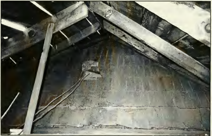
Figure 2.12a. Photo showing use of recycled materials. Building O, Rm. 5, East wall; tin can seal over knot holes. Photo taken 13 June, 1996 by P.D. Schulz.
