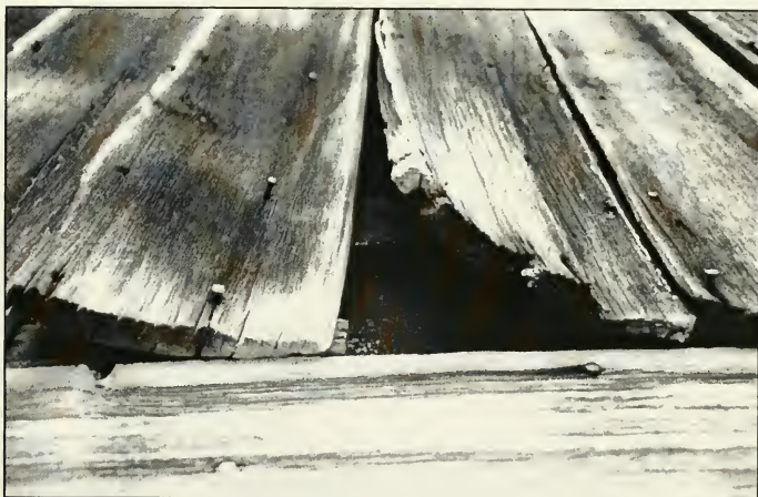
Figures 3.11a & 3.11b. Diagram and Photograph of types of material failure (physical). Photograph of South Elevation siding west of Win. 3, Building "N." Taken 14 June, 1996 by P. D. Schulz.
