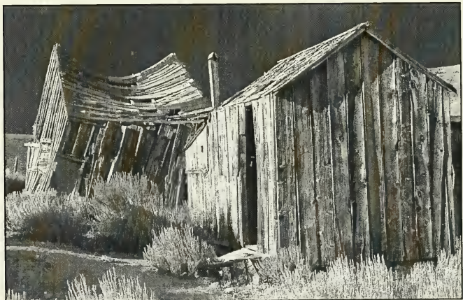
Figure 3.7a. Diagram of failures due to loads in gable roof. Rafters act as an arch. Figure 3.7b. Photograph illustrating deformation of structure into trapezoid. Members buckle due to lack of ridge member and collar ties. Lester Bell House Barn, looking North. Photo taken 3 Sept., 1998 by A.S. Morrison.
