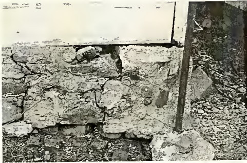
Fig. 2. The character of the masonry is fieldstone with some granite. It is pulling apart at the corners.
