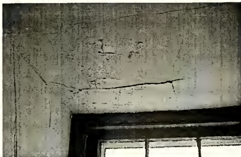
Fig. 9. Water damage above the dormer.
