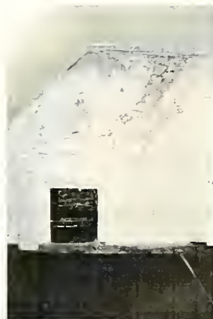
Fig. 14. Water damage on the third floor.
