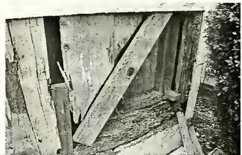
Fig. 1. Exposed rotted framing on the middle building.
