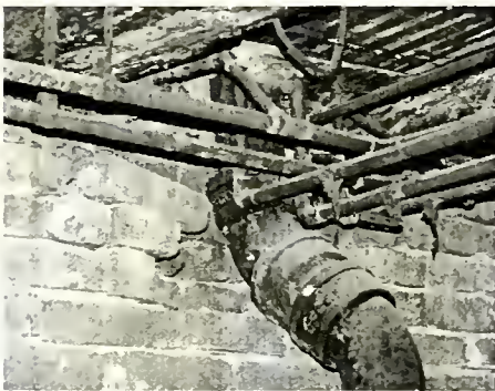
Fig. 4 & 5. Plumber damage in the basement.
