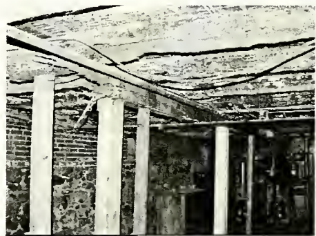
Fig. 1. The quasi-summer beam and some evidence of termite damage.
