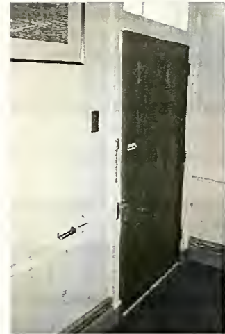
Fig. 6. The warp in the front door is evident.
