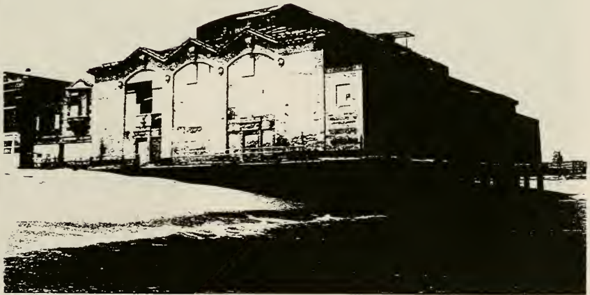
Ill. 69. View of deteriorated Casino Arena, 1996.
