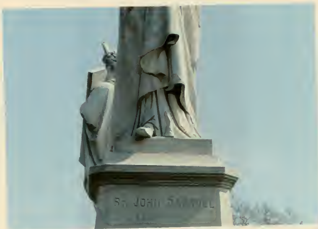
Figure 33: Gypsum crusts in undercut areas where rainwater does not regularly wash (Photograph by author, March 2002)
