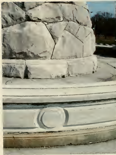
Figure 27: Cracks and invasive vegetation in concrete bed of the basin
