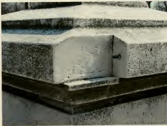
Figure 26: Missing dutchman repair and exposed metal pin
