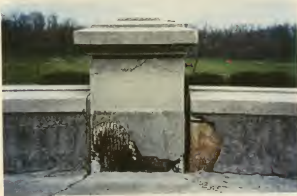
Figure 24: Open joints and mortar loss in the basin wall
