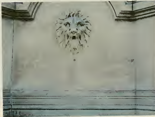
Figure 28: Evidence of inappropriately removed graffiti from pedestal
