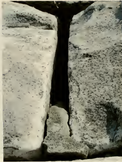
Figure 17: Loose and missing mortar from a joint in the rock mound base
