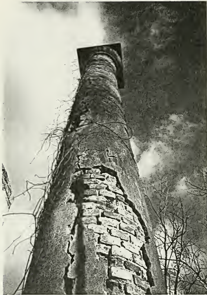
Figure 37: Typical column deterioration
