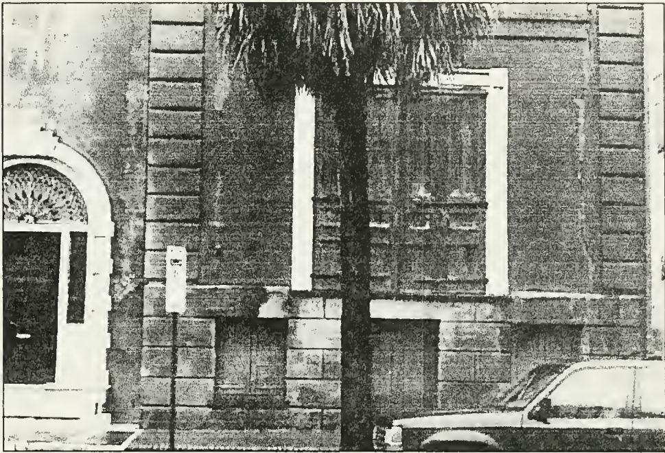
Figure 4.4. Cementitious composites used to patch original stucco may provide a temporary cure for unsightly cracks which result from structural inefficiency, but may also damage existing historic fabric. West facade.
