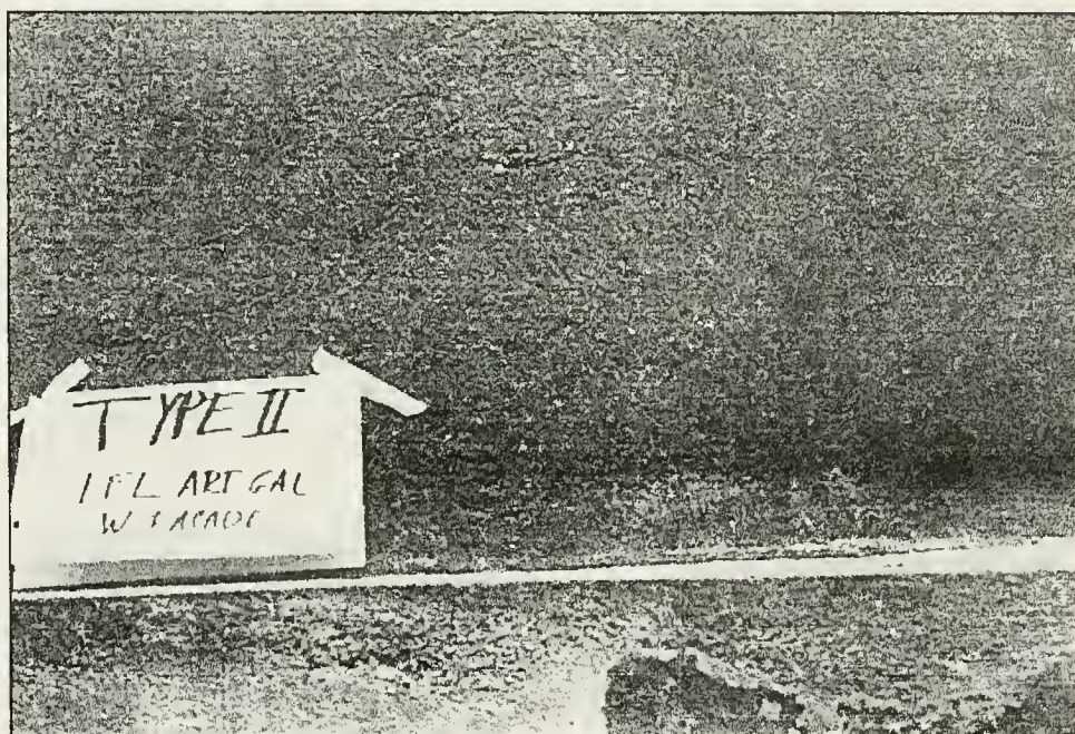
Figure 3.8. Example of stucco type 2, applied to exterior surface of 1858 art gallery. Visually and presumably compositionally different from type 1, it is characterized by floating tool marks applied in a circular pattern. West facade, first floor of art gallery.
