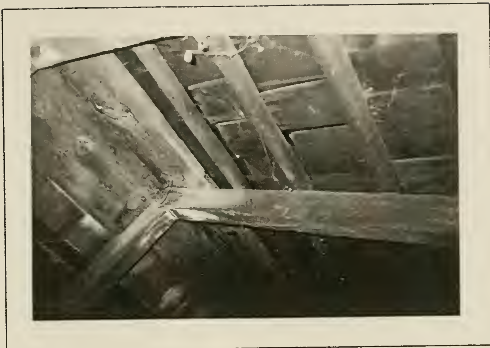
Plate 67: View into roof space above attic, 1991. Note wood shingle roofing in place below current standing seam metal roof.
