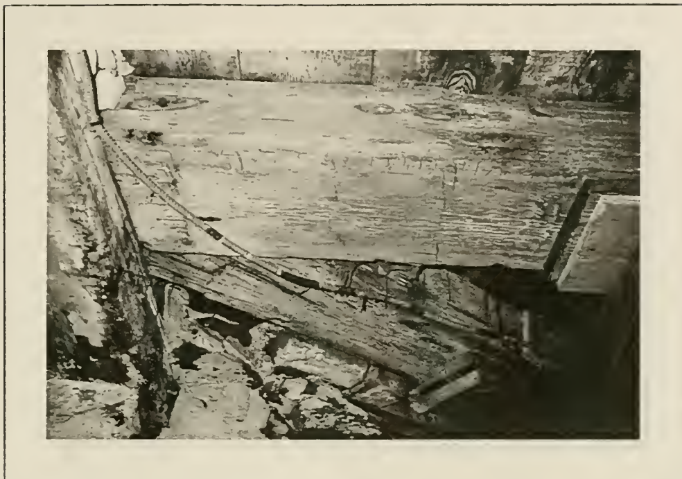
Plate 33: Detail of first floor joists bearing on lintel of basement stair opening, 1991. Note diagonal header below corner fireplace above.
