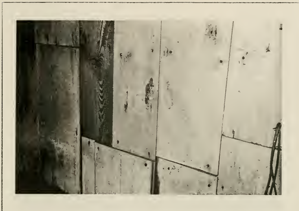
Plate 65: Detail of board partition at attic stair, 1991. Boards reused from Rm.202 partition.
