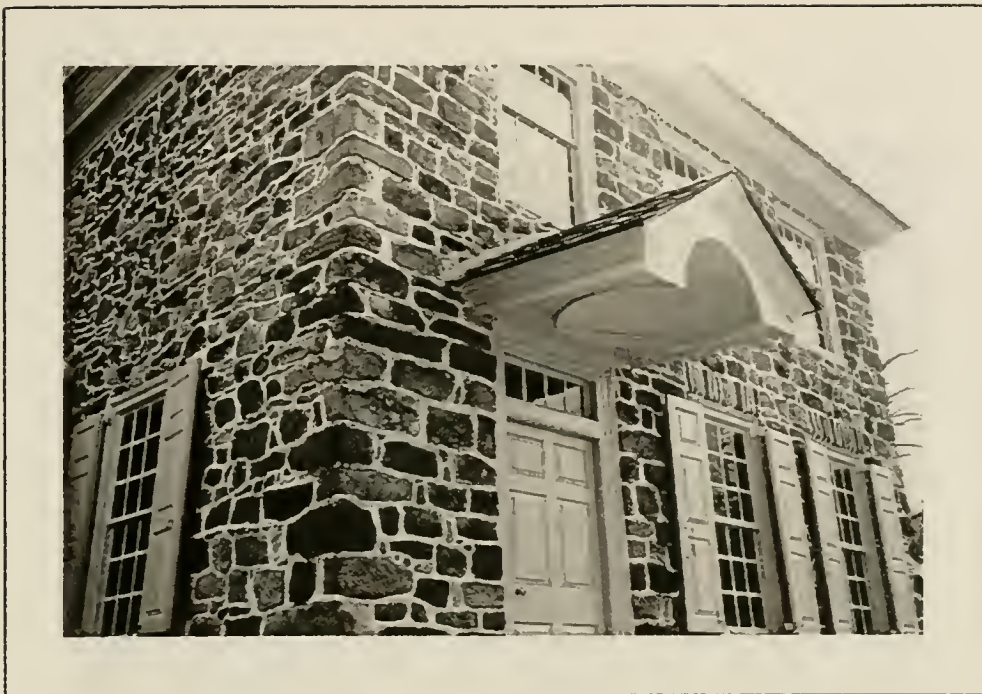
Plate 77: View of southwest corner of Isaac Potts House, 1991. Note differences in masonry.
