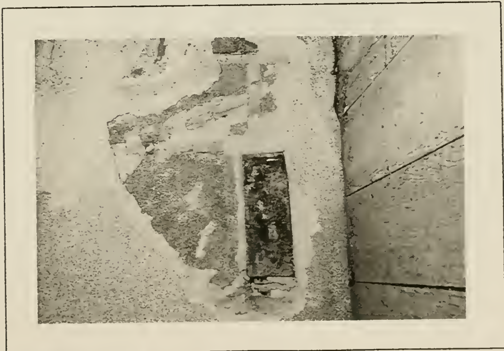
Plate 19: Detail of surviving mortar flashing of door hood above north entry door, 1991.
