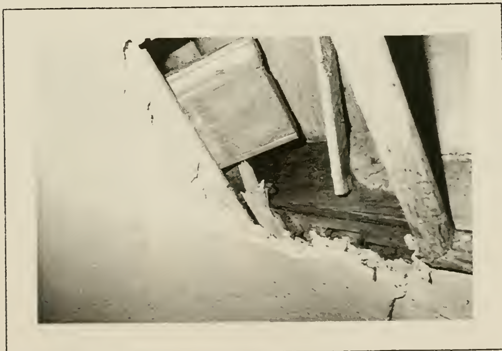
Plate 68: Detail of late 18th century jamb molding found in attic reused as nailer behind 19th century ceiling, 1991.
