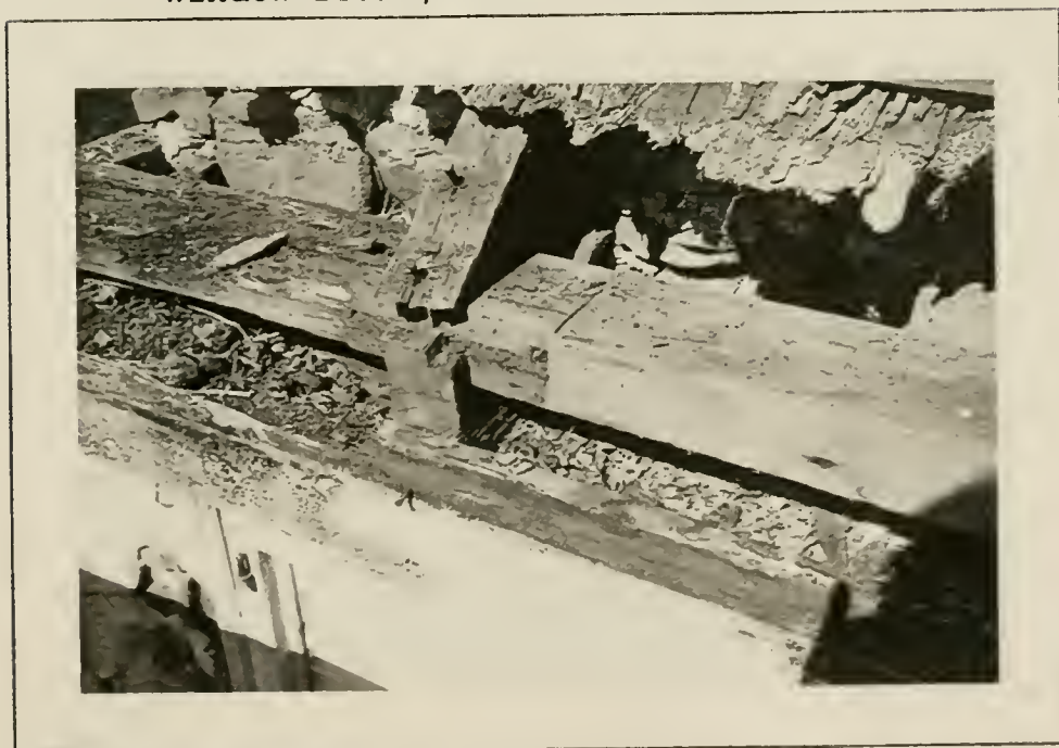
Plate 26: Detail of cornice framing, east side, 1991. Note rafter tips, plate and floor joists.
