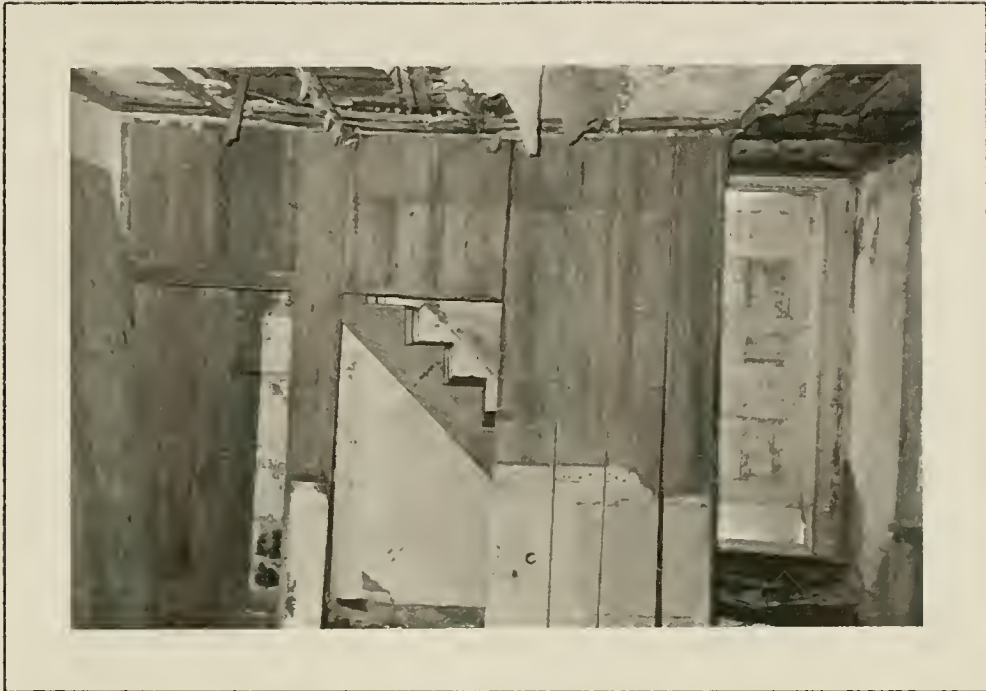
Plate 42: View of beaded-board wall at stair in Rm.102, 1991. Door at right cut through masonry in 1950s, center door in board wall circa 1880, door at left to cellar stair circa 1836..
