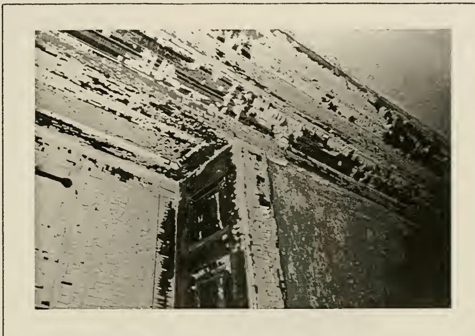
Plate 35: Detail of wood cornice and panelled door jamb at entry door to Rm.101, 1991.
