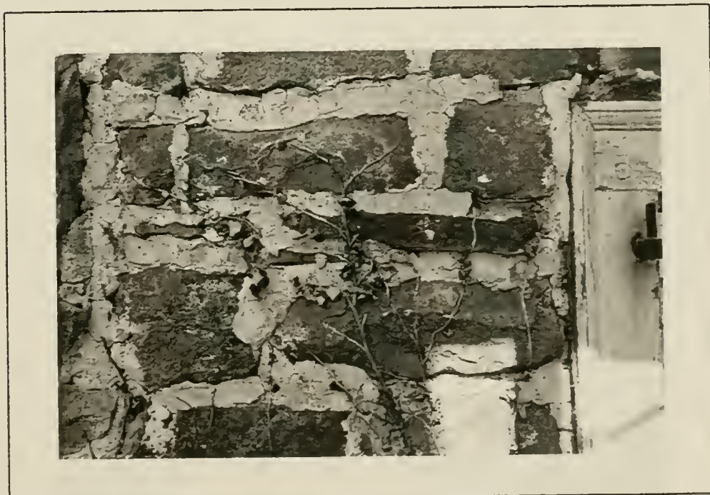
Plate 24: Detail of surviving smear pointing at first floor level of east facade, 1991.
