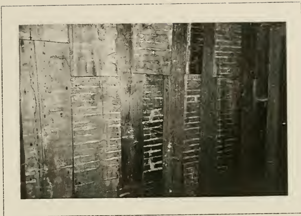
Plate 63: Detail of partition at attic floor level with plaster and lath removed.
