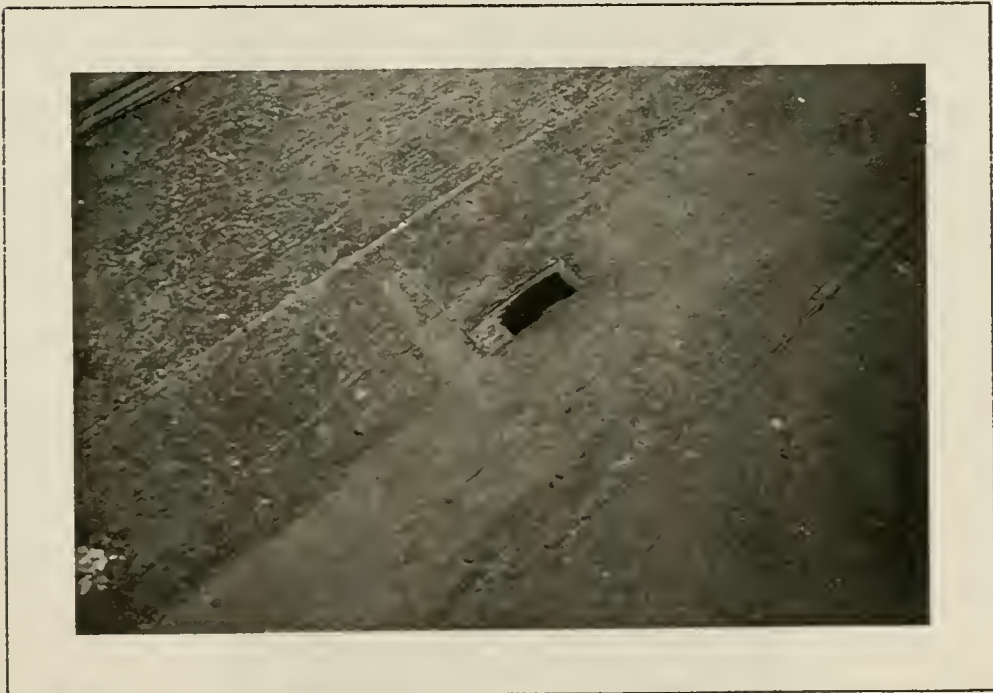
Plate 50: Detail of imprint on floor of 18th century partition and door jamb at top of stair on second floor, 1991.
