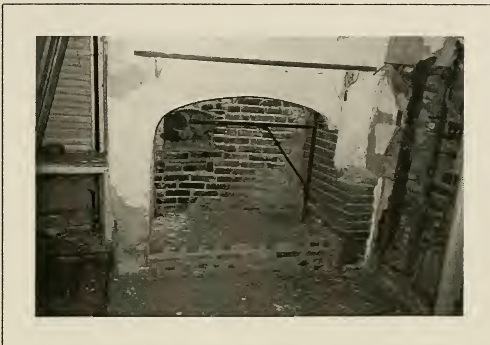
Plate 40: Detail of 19th century cooking hearth in Rm.102, 1991. Note location of oven door.
