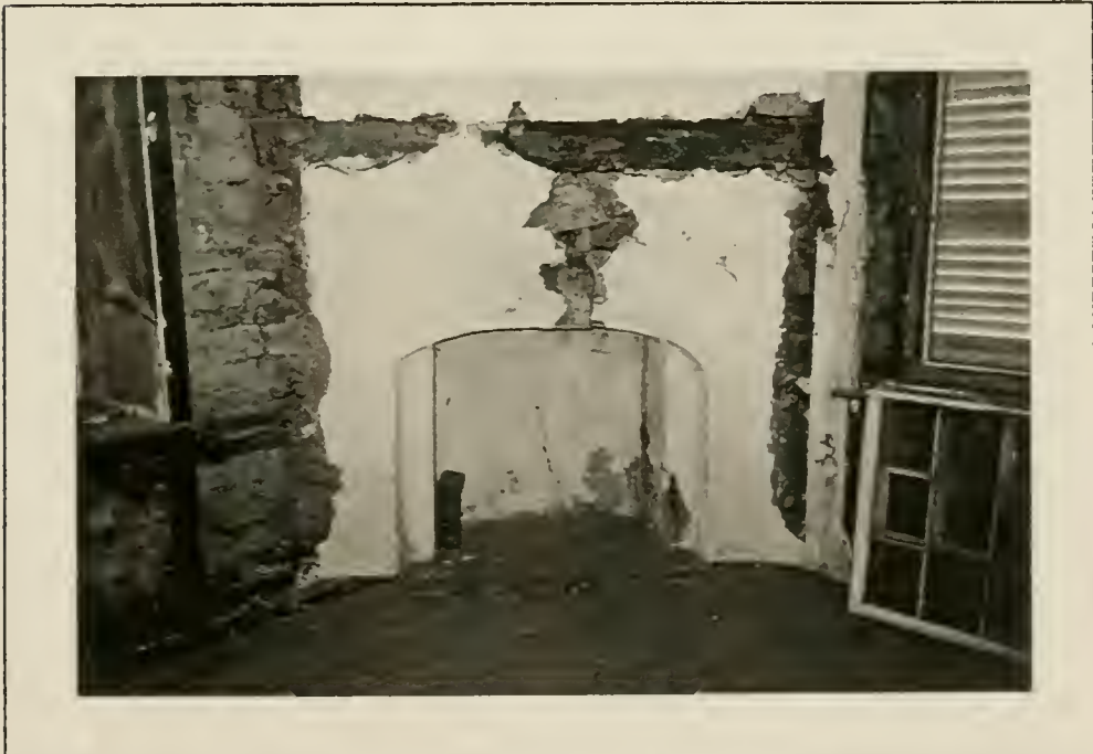
Plate 56: Detail of corner fireplace in Rm.202, 1991. Note evidence of baseboard and chair rail.
