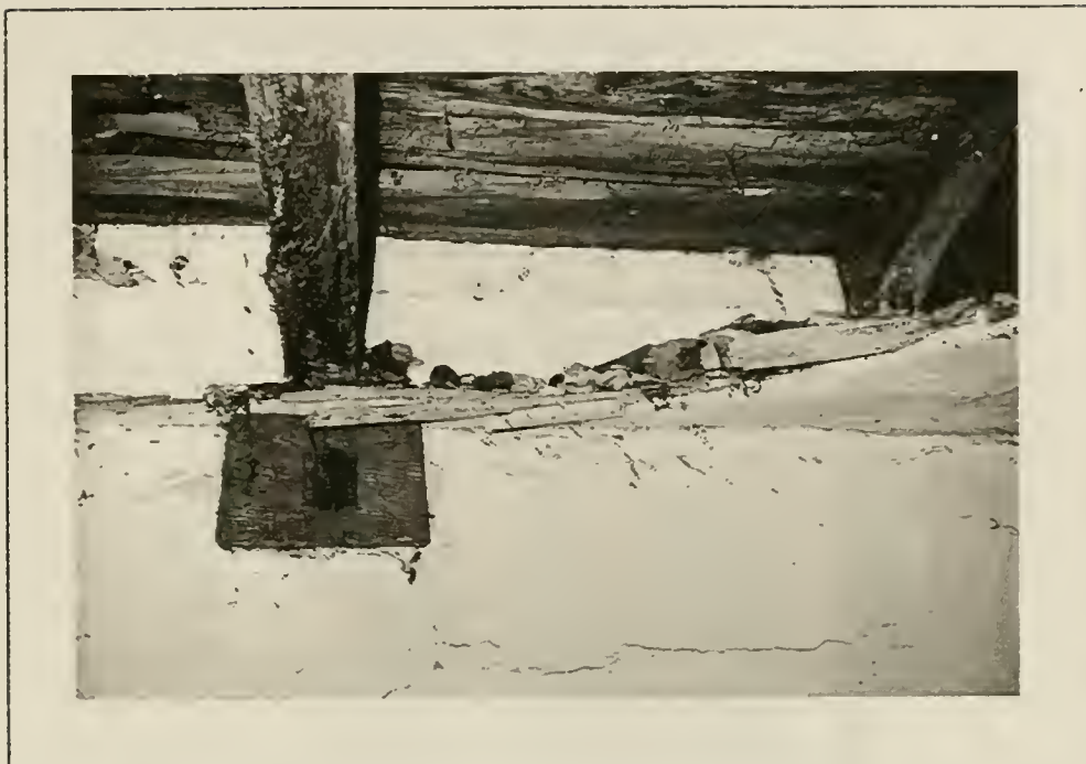
Plate 57: Detail of 18th century wall plaster in place above 19th century ceiling on west wall of Rm.202, 1991. Joists were originally exposed.
