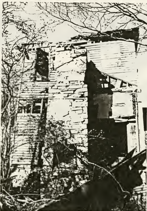
Figure 90: Damage to East Elevation of Federal Main Massing
