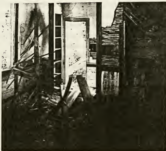
Figure 92: Collapsed Floor of Federal East Parlor (Foreground)
