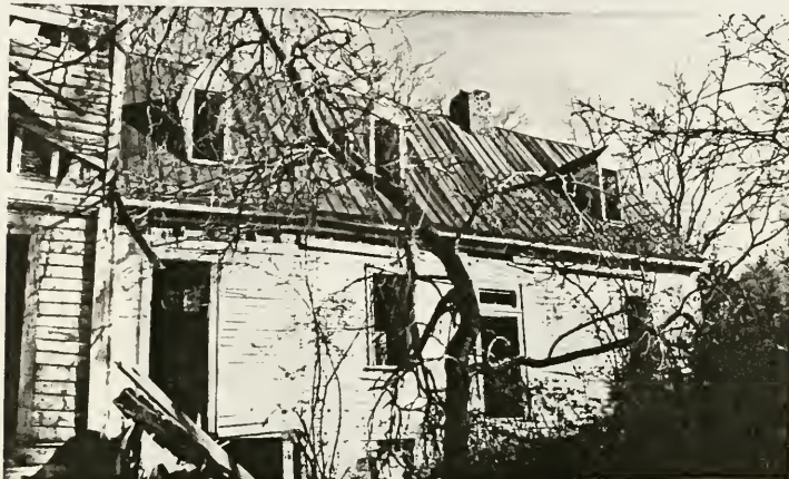
Figure 88: Damage to West Elevation of Georgian/cross hall section
