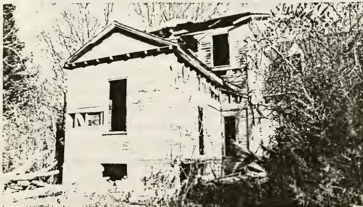
Figure 89: Damage to Federal West Elevation
