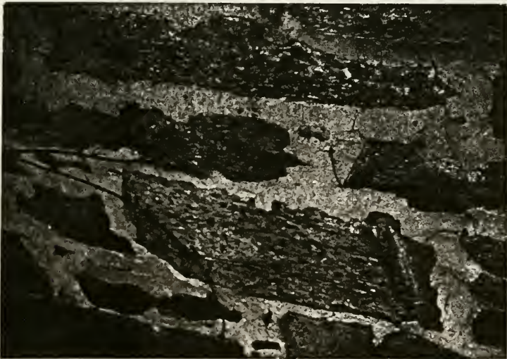
Figure 10: Gneiss Foundation Below Main Door of North Elevation
