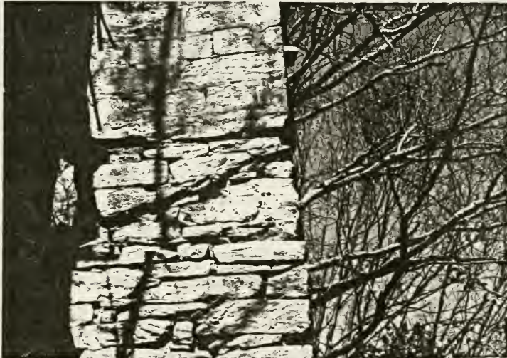
Figure 82: Ghost Mark of Front Gable Roof on South Elevation of Federal East Chimney
