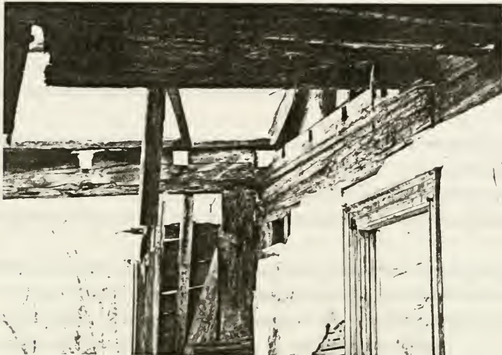
Figure 91: Damaged Roof Near East Elevation of Federal Main Massing
