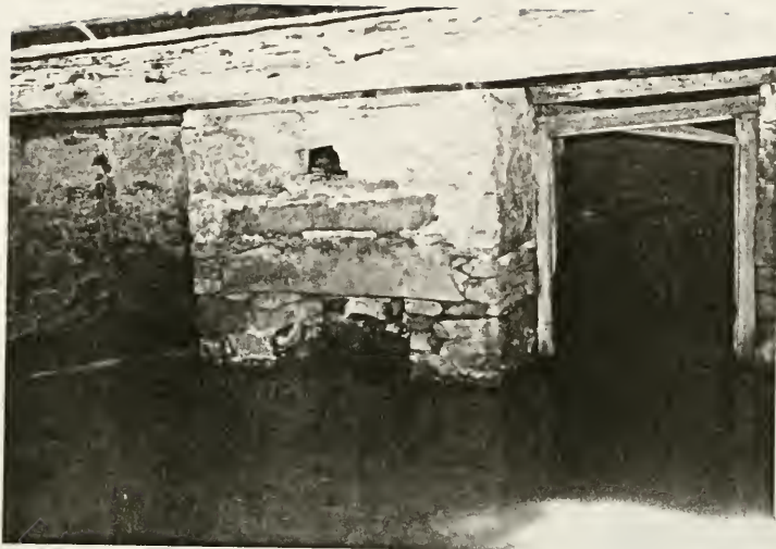
Figure 86: Flooded Basement under Georgian Parlor
