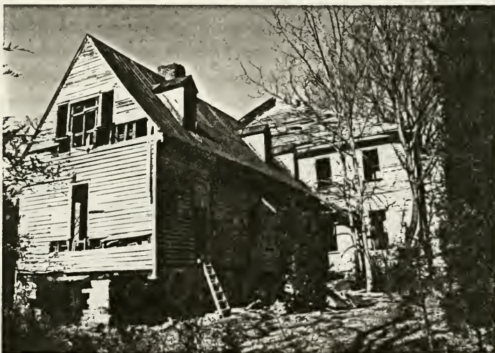
Figure 85: Loss of Fabric at Southeast Corner of Georgian/cross hall Section
