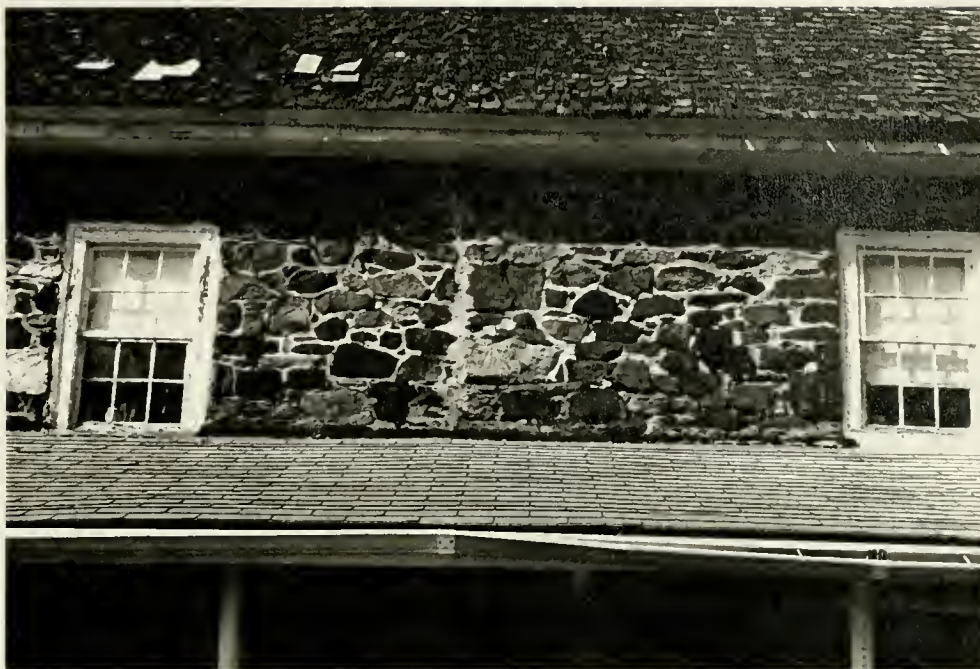
Fig. 3.11. Regester -Black House. Detail of vertical and horizontal seams. South facade.
