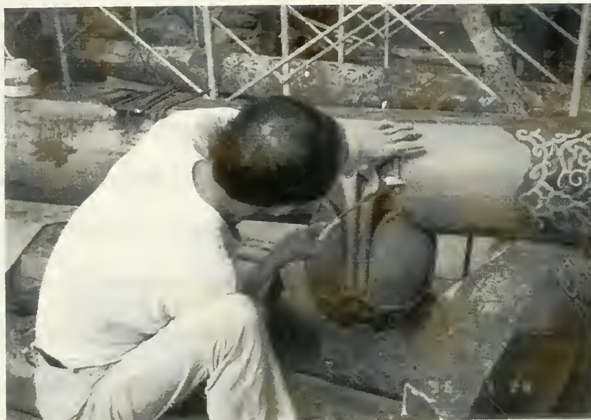
Fig. 4.3 A craftsman was filling the missing part of a wooden component (photographed by the author)
