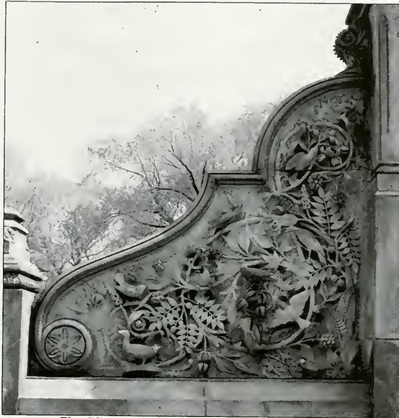
Fig. 28 - Northwest bird panel, western exposure. Note erosion under drip molding along the top.
