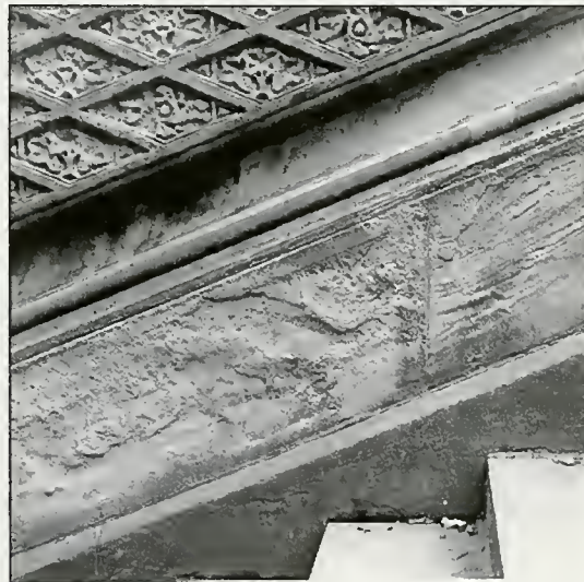
Fig. 6 - Retroweathering - retroweathering on wall panel base of north arcade stair.
