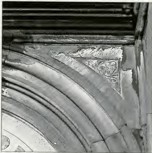
Fig. 18 - (2c.a) Efflorescence - loose salt deposits on stone surface.
