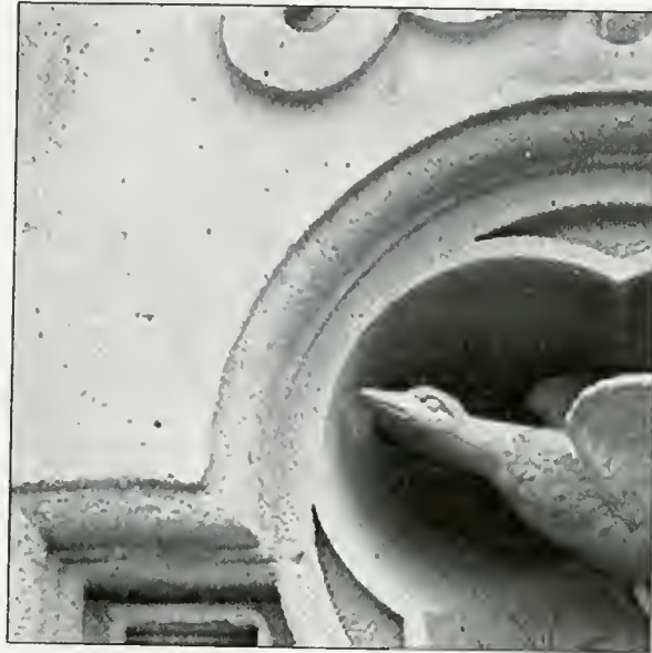
Fig. 11 - (1b.g) Pitting – alteration of stone surface resulting in pitted areas where less stable components weather out of the stone.
