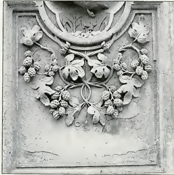
Fig. 23 - (3f.b) Delamination - detachment of larger stone elements parallel to stone structure, but not necessarily to stone surface.
