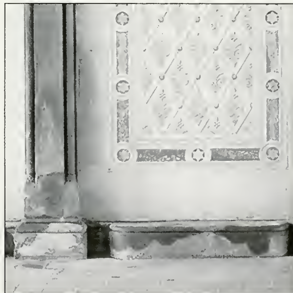
Fig. 16 - (2b.b) Soiling from ground water - often the result of rising damp and water penetration.
