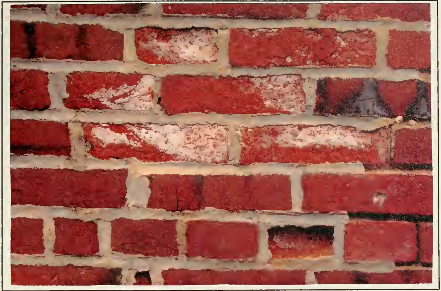
Figure 6 Efflorescence on nineteenth century hand moulded brick. Note the inappropriate repointing which can be a cause of extrinsic soluble salts.
