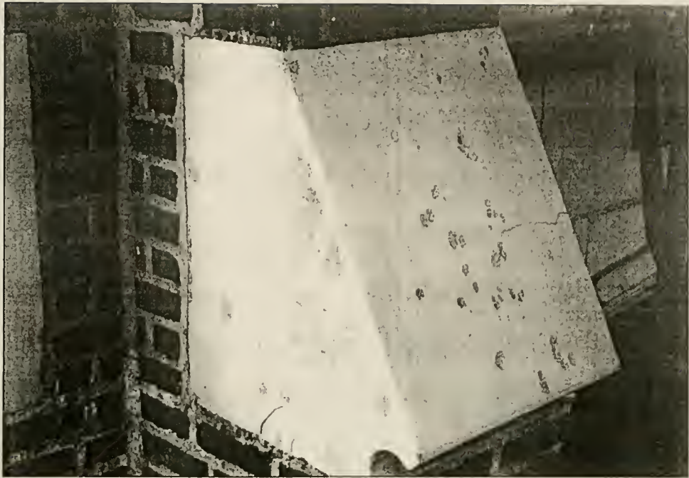
Figure 3.2 Glaze spalling, Ventnor City Hall, Ventnor, New Jersey (Vivian Smith, 1928-29).
