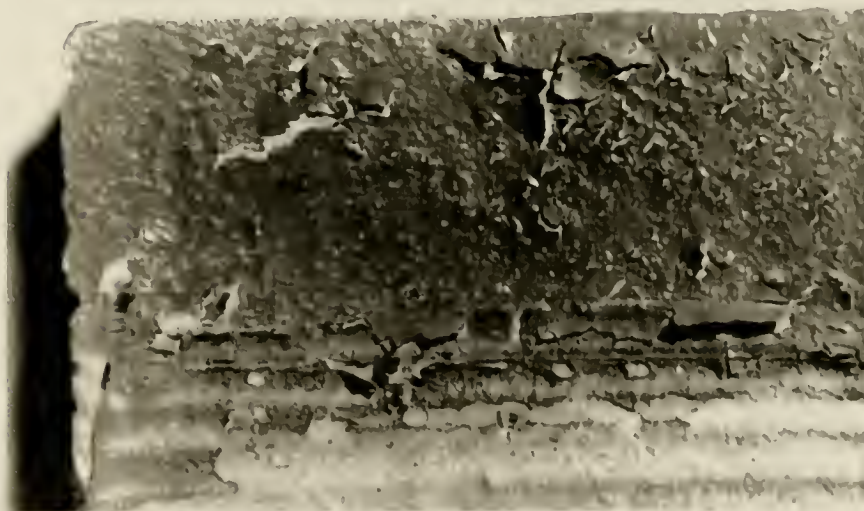
Figure B.23 Edison Aquathane UA-210-H specimen 1B mortar after 52 cycles. Note excessive map cracking, mortar exposure, and coating peeled from glaze surface.
