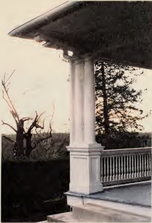
Figure 54. Detail of east end of porch showing the Colonial Revival scroll bracket. (1994)
