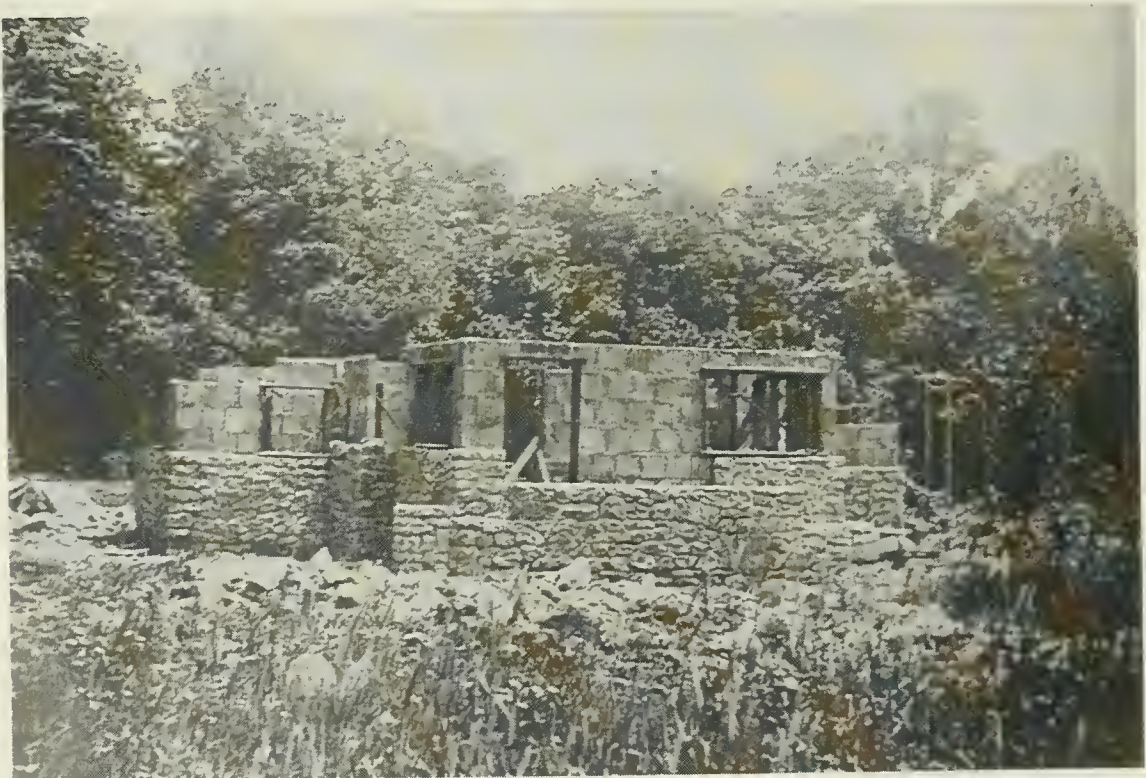
Plate 54. Rest Cottage. Under construction, 1910. This view of the southwest corner of the house shows the hollow tile construction method utilized by Price. This dwelling was designed by William Price and constructed following Joseph Fels' plea for more permanent architecture to be built in Arden. This house was built of hollow tile and plaster with a rough stone foundation. Courtesy Peg Aumack.
