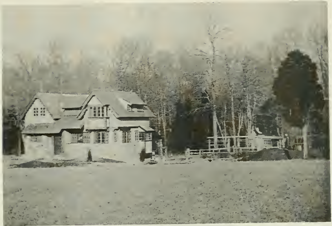
Plate 39. Second Homestead. Under construction in 1909. This view shows the hollow tile used in the construction of this dwelling. Courtesy Peg Aumack.
