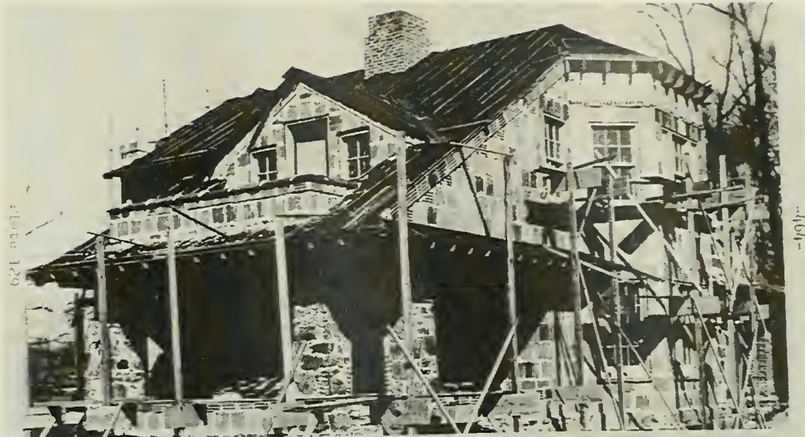
Price and McLanahan: Rose Valley Improvement Company Houses, Rose Valley, Pa. 1910 - 1911. House during construction.
