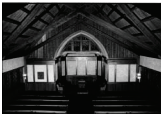
Sanctuary and apse before rehabilitation.
