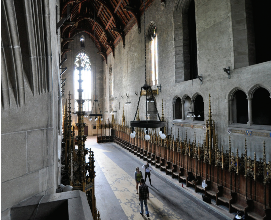
Figure 21: St. Andrew's Chapel "View of sanctuary from above showing the existing plywood floor" (photo courtesy of The University of Pennsylvania Graduate Program in Historic Preservation, fall 2010)
