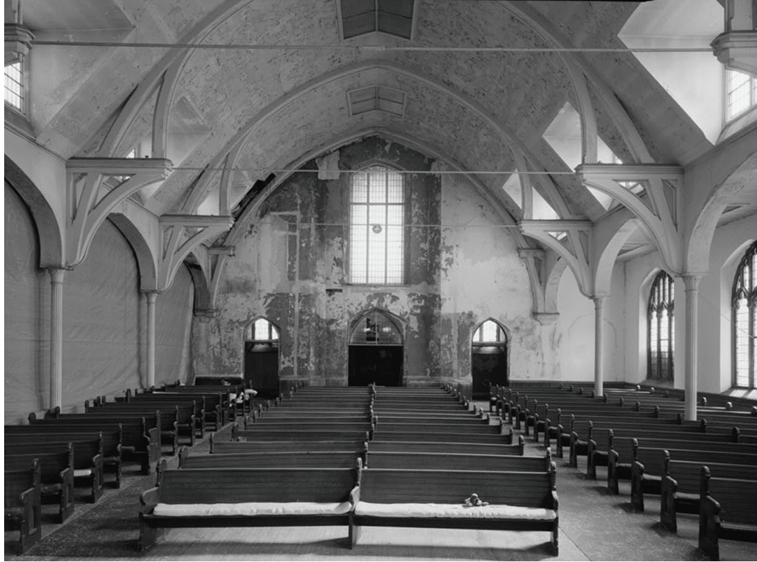
Figure 3: Green Hill Presbyterian Church: rafters with iron tie rods, Philadelphia (Demolished) (Photo courtesy of Library of Congress, Prints & Photographs Division, HABS PA,51-PHILA,741-7, documentation compiled after 1933)
