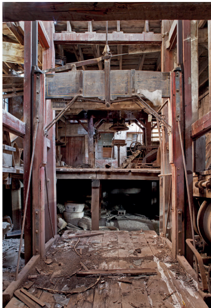
Figure 2.39: Two-story tile shop lift at Wester Clay. Joe E. B. Elliott, photographer, July 2011. Courtesy of the University of Pennsylvania Architecture Conservation Laboratory.
