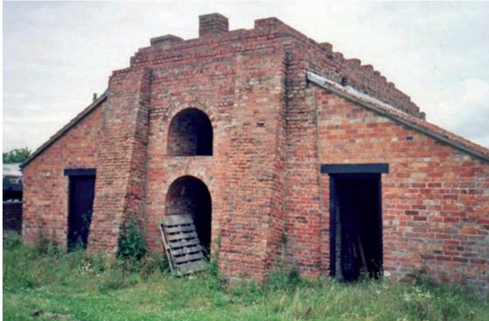
Figure 2.14: Modified version of a Scotch Kiln. "Baumber Brick Kiln." Ken Redmore, photographer, 2006. Society for Lincolnshier History and Archaeology. Image from http://slha.org.uk/slha/Main/GalleryBricks .
